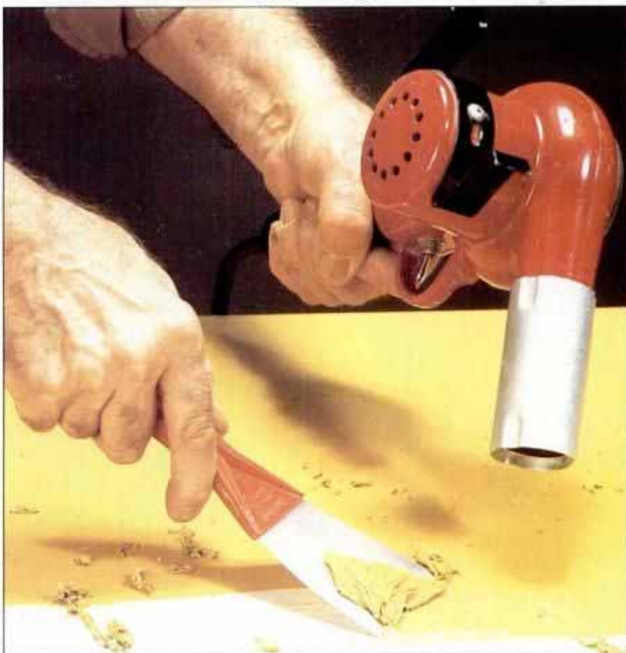
One of the best ways to remove layers of old paint is with a heat gun and putty knife.
