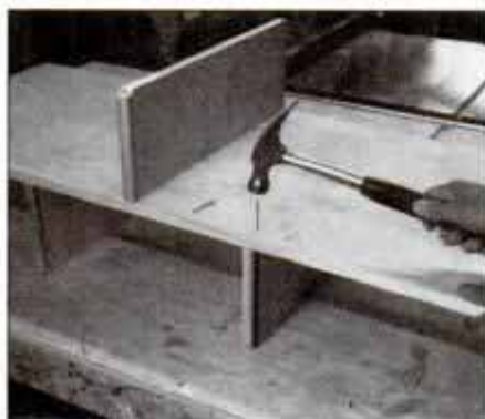
5 Install the partitions in the dados with glue and 6d finishing nails. Use four nails per joint and make sure the edges are flush.
