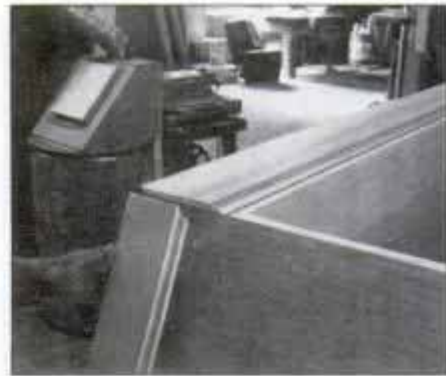
14 The long front trim piece is installed first. Then, miter the end trim pieces, cut to length and glue and nail in place.
