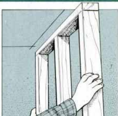
3 Prior to cutting the center joist, erect temporary 2x4 support partitions about 3 in. away from each rough opening end.
