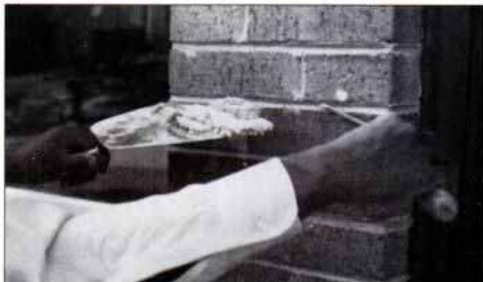
Dampen the joints, then apply new mortar using a mason's trowel and a narrow joint filling tool as shown above.
