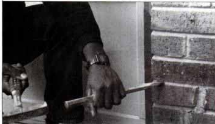
To repoint brickwork, begin by removing the old mortar. Use a 1/2-in. cold chisel and mason's or ballpeen hammer.
