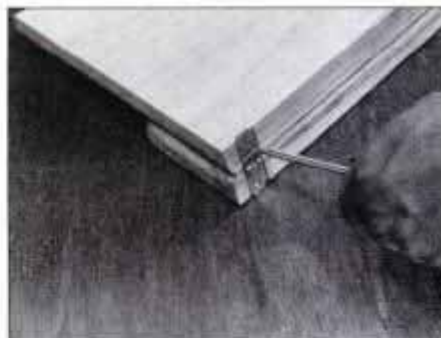
13 Use a fine back saw and sharp chisel to cut the hinge mortises. Then, bore pilot holes and screw the hinges in place.
