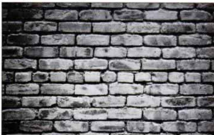
This brick wall shows the effects of moisture damage. As the water freezes and thaws with the change of seasons, it expands and contracts which ends up cracking the mortar and the bricks.
