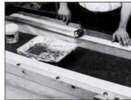
6 Prepare 1 pound of plastic resin glue for each laminated slat. Apply a uniform coat to parts with a 3-in. paint roller.
