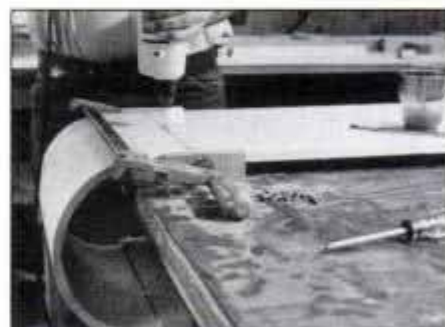
15 Clamp each cleat in place and bore pilot holes for the 1-in. No. 12 solid brass screws. Countersink \frac{1}{16} in. below surface.
