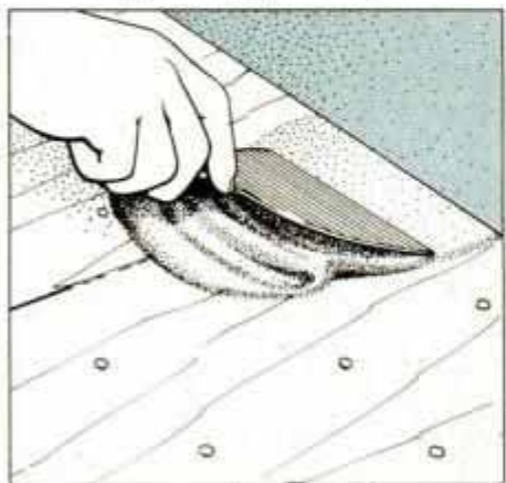
7 Set nailheads below surface. Fill holes and seams with patching compound. Let dry and sand smooth with 100-grit paper.
