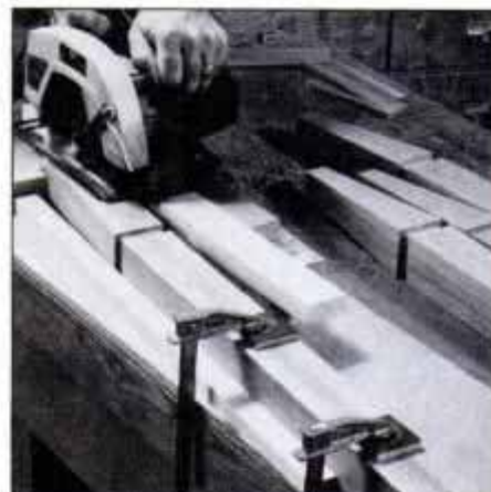
3 Circular saw rides on a 2\frac{7}{16} -in. ledge spaced at the appropriate line of cut. Rotate the stock after each pass.
