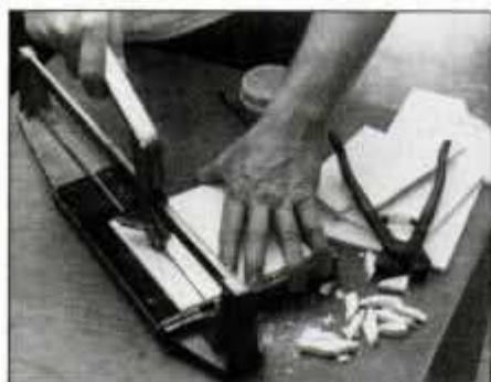
Tile cutter requires running over tile a couple of times to score glazing, then pressing down on handle to break or snap tile.
