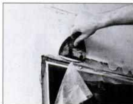
Fill all minor cracks and depressions with joint compound. Deeper holes require patching plaster first, then compound.
