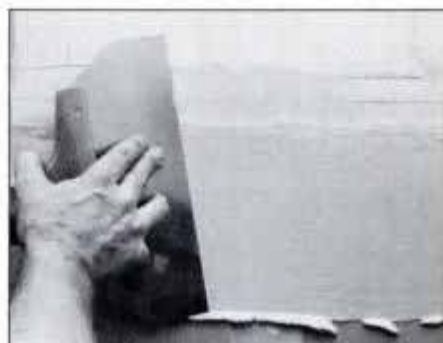
Apply self-adhesive fiberglass mesh tape over joint and cover with joint compound. When dry, apply a second coat.
