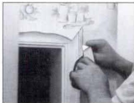
Cut wallpaper corner back at angle to permit fitting neatly along the door frame casing molding. Don't stretch the paper.
