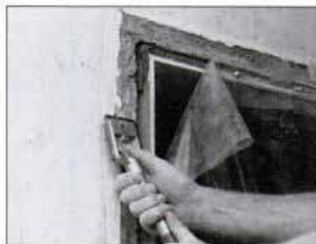
Scrape off all old paint build-up and loose plaster using hand scrapers. Cover doorways to prevent dirt and dust from spreading.
