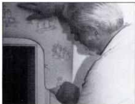
Cut away excess wallpaper leaving 2- to 3-in. allowance for trimming. Note the rounded corner is less likely to tear when wet.
