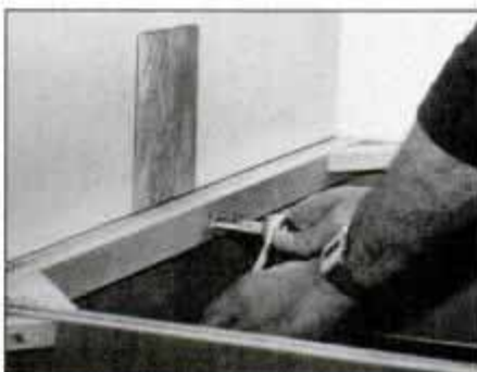
Fasten base cabinets to studs with lagscrews—or toggle bolts, if no stud can be found. Shim cabinet back if wall is not straight.
