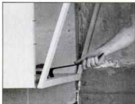
Remove old cabinets first. Use a flat pry bar or wrecking bar to pry off face frames. Then remove the bottom, sides and tops.
