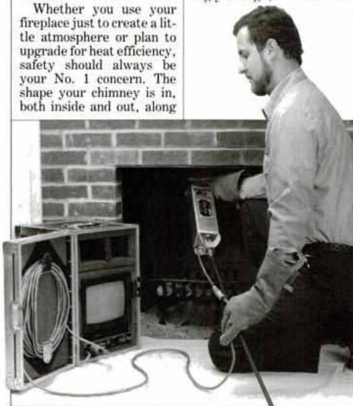
One great way to check the chimney's creosote build-up is with video scanning equipment, operated by a certified chimney sweep.
