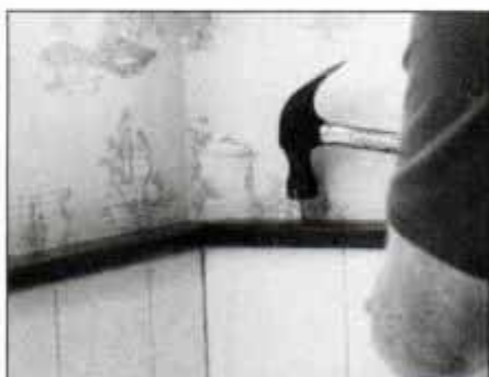
Install trim—in this case prefinished cherry boards—to backsplash. Use glue and finishing nails. Set and fill all nailhead holes.
