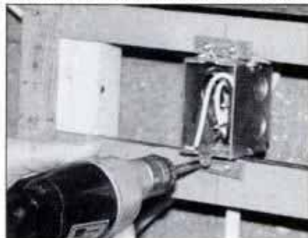
Plan location of all outlets carefully. It's much easier for the electrician to run these lines when the inside of the wall is accessible.
