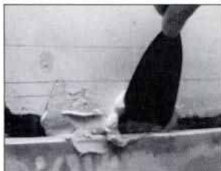
Fill all joint gaps with plaster to within ¼ in. of surface. Smooth with a wide joint knife and let the plaster dry thoroughly.
