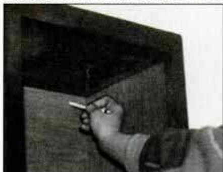
Prebore holes for stud locations in the back of the wall cabinets. Then lift into place and attach with lagscrews and washers.
