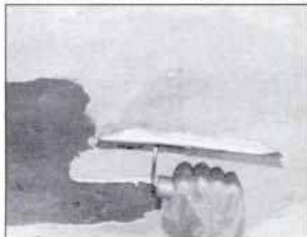
First, chisel off all loose plaster from ceiling, then fill with patching plaster to ¼ in. of surface. Finish with joint compound.
