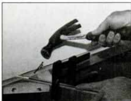
Toenail rear of base cabinets together with 6d finishing nails. Clamp and use thin spacers between cabinets, if necessary.
