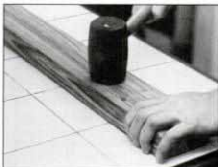
Use flat wood block to span four to six tiles. Then tap board lightly with a rubber mallet to seat the tiles uniformly in the mastic.
