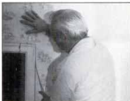
After fitting the top edge of strip, adhere rest of wallpaper following plumb line previously marked on wall for right edge guide.
