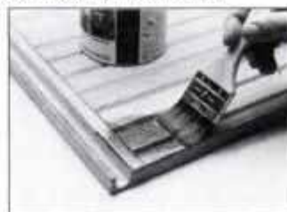
Finally, apply a finish such as stain, paint or varnish. Note the continuous pull on door end.
