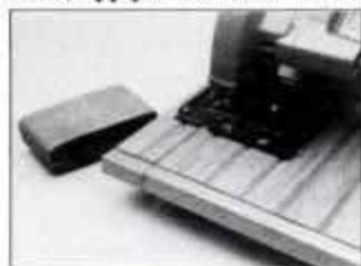
To make custom-fit doors, first rip the door to desired width using a portable circular saw.
