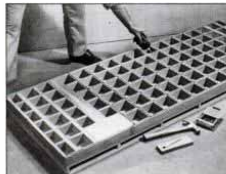
8 After one side of the eggcrate is stapled together, check for square, and apply slow-setting hide glue on all edges.
