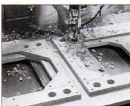
11 Cut the clamp access holes in the inner guides by first boring 1 1/2-in. holes and cutting the waste with a sabre saw.
