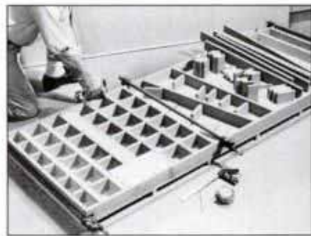
6 Hold benchtop components in place with pipe clamps and drive one staple at each web joint. No glue is needed.
