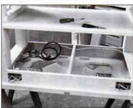
12 Mount the switch and outlet boxes on the long apron. An octagon junction box splits the circuit to the two tools.
