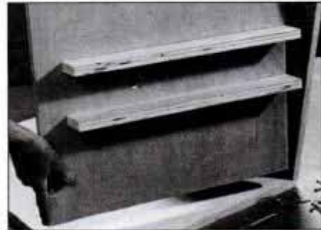
3 Before attaching the partition to the cabinet, bore a 1-in.-dia. bolt access hole and attach two plywood post guide strips.
