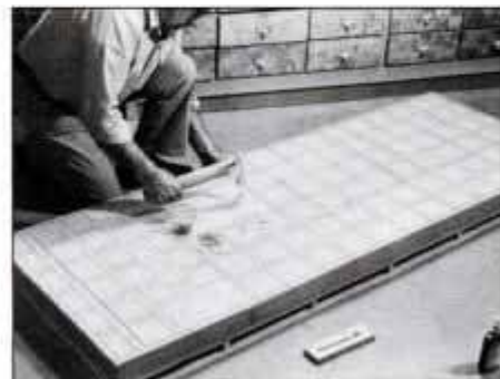
9 Instead of using clamps to hold the panel in place while the glue sets, drive finishing nails between each intersection.
