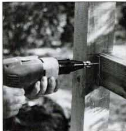
6 Place a 2x4 rail in the bracket and bore pilot holes to prevent splitting. Then, fasten the rail with ¼-in. galvanized screws.
