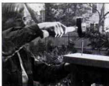
12 Top off the fence with a 2x6 cap rail. Fasten the rail with 20d (4-in.) galvanized nails. Space the nails about 24 in. apart.
