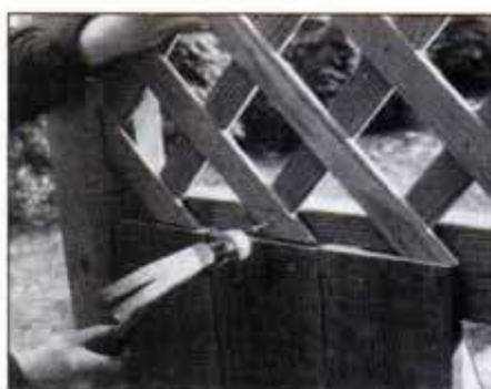
9 Bore pilot holes to prevent splitting the lattice. Then, attach it to the rails and 2x2 nailers with 4d galvanized finishing nails.
