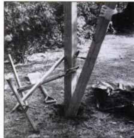
3 Backfill around the post and tamp the soil with a spare 2x4 rail. Continue to add soil and tamp until it's level with the lawn.
