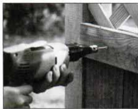
10 Use 1x4 trim to conceal the joint where lattice meets 1x6 boards. Fasten 1x4 trim with 2½-in. galvanized screws.
