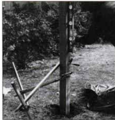
2 Support the post in the hole with two diagonal braces clamped to stakes driven in the ground. Use a level to plumb post.
