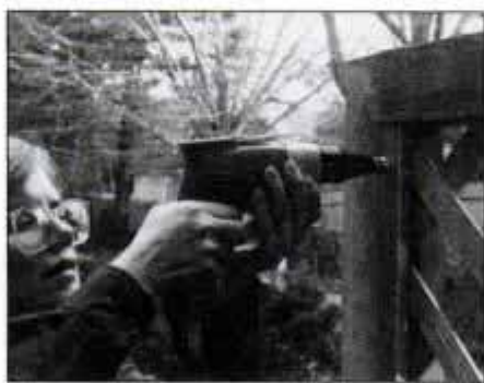
11 Attach vertical 1x2 trim at the ends of the lattice panels with 2-in. screws. Bore pilot holes first to avoid splitting the trim.
