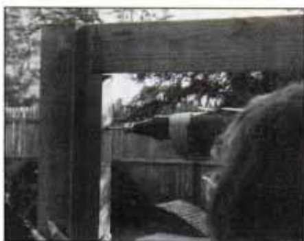
8 Attach 2x2 nailer strips to the fence posts with 2½-in. screws. The strips provide a solid surface for fastening the lattice.
