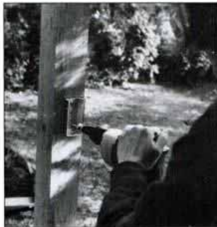
5 Mount brackets to posts with ¼-in. galvanized screws. Electric screwgun provides no-sweat way to drive screws.
