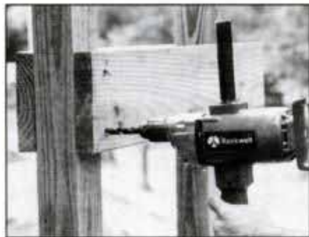
10 Tack-nail ledgers for lower deck to both sides of posts. Then bore clearance holes through parts for carriage bolts.
