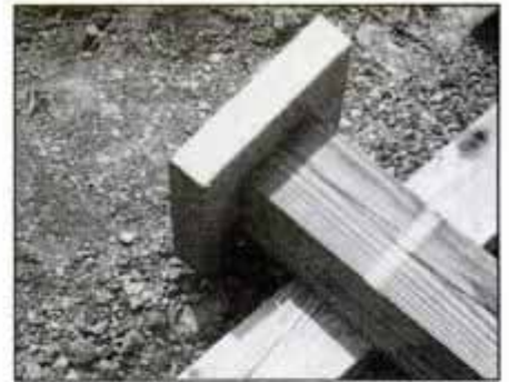
3 Dig holes at proper locations, then nail a 2 x 8 block to the bottom of each 4 x 4 post. The blocks help distribute deck weight.
