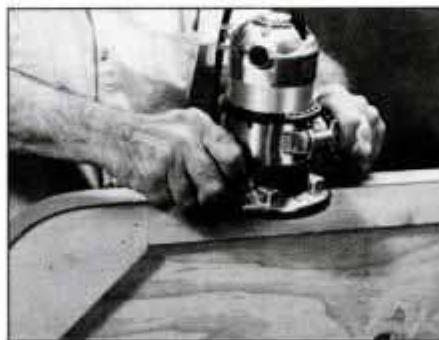
Trim off the overhanging edges of the laminate with a router fitted with a flush-trimming bit. Be sure to wear goggles.
