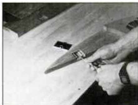
7 Mark hinge positions and use a sharp chisel to cut each hinge mortise. Note extra recess required for hinge barrel.
