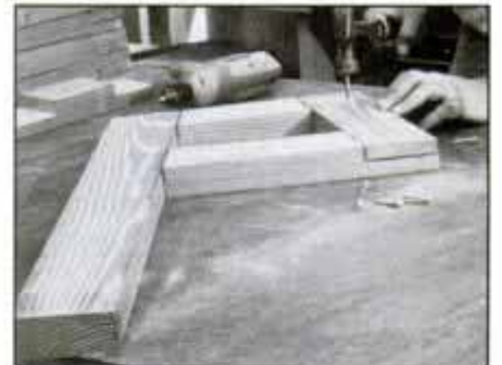
21 Cut bench support parts to size, then cut all required half-lap joints. Join with plastic resin glue and galvanized nails.
