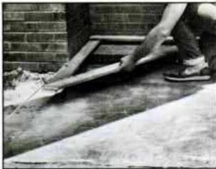
1 Lay out perimeter of deck using mason's string and batter boards. Check corners for square with 3 x 4 x 5-ft. triangle.
