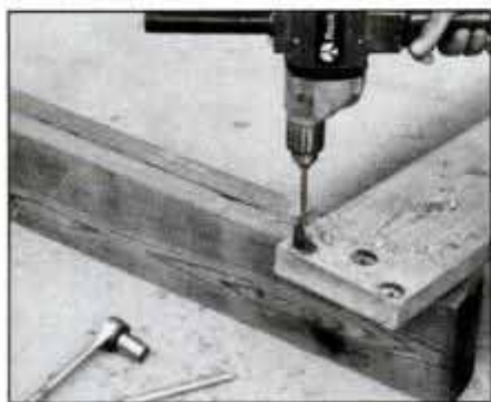
7 Remove ledgers and bore pilot holes at end for lagscrews that hold double end joists. Counterbore to accept socket wrench.
