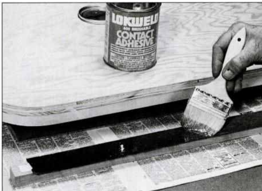
Apply contact cement to laminate and to the edge of core. When it's dry, apply a second coat. To brush on the contact cement neatly, tape the laminate strip to a narrow wood stick.
