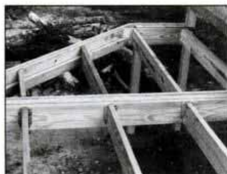
13 Install hangers, then cut joists to fit and nail in place. Ends of joists must be notched where they meet angled 2 x 4 ledgers.
