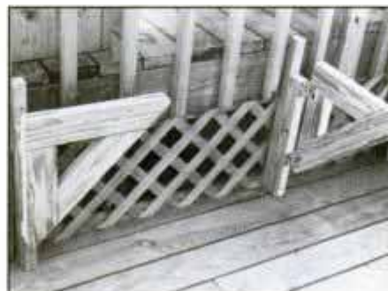
23 Cut parts for support braces on folding table to size and join with half-lap joints and hinges. Attach supports to deck framing.
