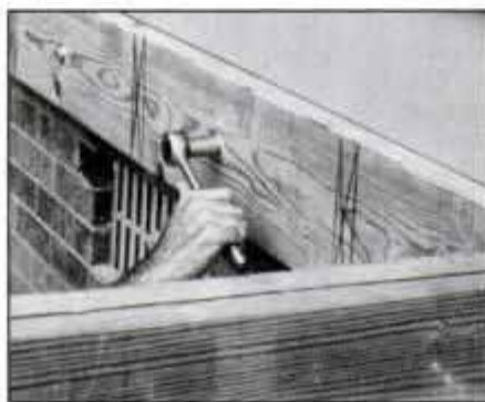
8 Attach ledger to end joists then support assembly and attach to house wall as a unit. Tighten ledger lagscrews securely.
