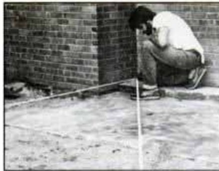
2 When all strings are in place, check for square by comparing diagonal measurements. The diagonals should be equal.
