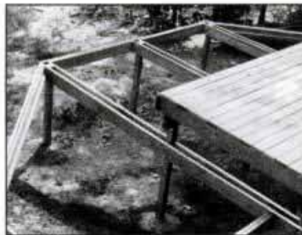
11 First install all ledger boards and facing boards on lower deck. Then lay out joist positions in center sections.
