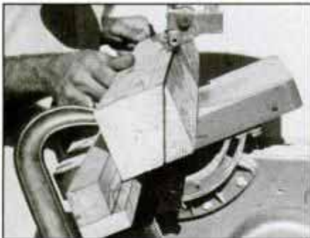
19 To form angled corner posts, rip 4 x 4 stock to 22\frac{1}{2}^\circ on band saw. Circular saw will work if cut is made from both sides.
