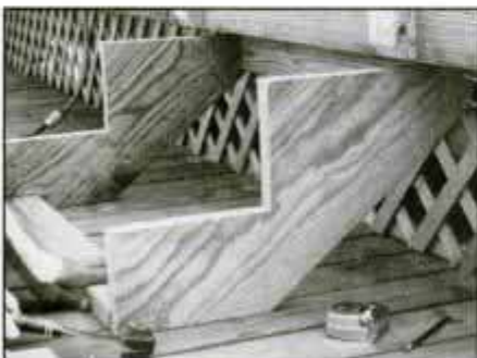
22 Nail 2 x 4 cleats to upper deck beam and lower deck floor boards. Cut stair stringers to shape and nail into cleats.
