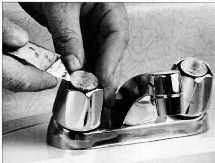
1 Begin repair by removing decorative caps from handles using a utility knife. If your faucets don't have caps, look for a setscrew at the bottom of the handles.
