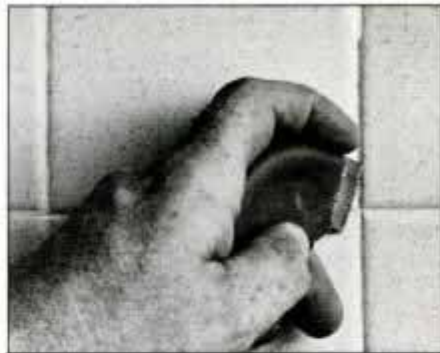
1 Begin repair by digging old cracked grout from joints using grout removal tool. Clean out to a depth of at least 1/16 in.
