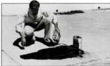
To use FADE, just pour it on an oil stain and let it soak to penetrate the concrete.
