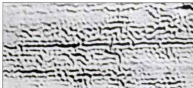
Wrinkling is caused by paint that doesn't dry properly.
