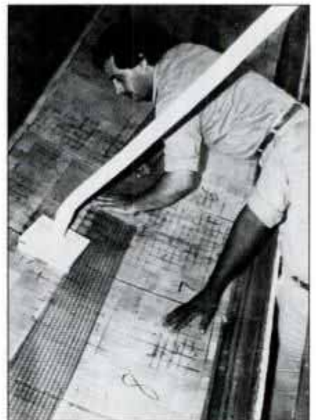
Vacuum pipe removes air from beneath plastic sheet, creating a uniform bond.
