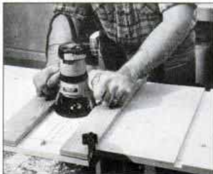
5 Rout dados for the shelves in the cabinet sides with \frac{3}{8} -in.-dia. straight bit. Parallel straightedge guides ensure accurate cuts.
