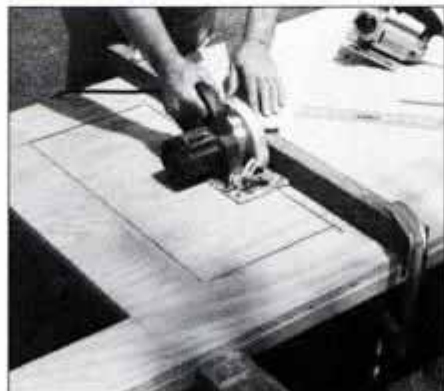
Then, lower saw slowly until it sits flat. Advance saw along the fence to the corner. Reposition fence for the remaining cuts.
