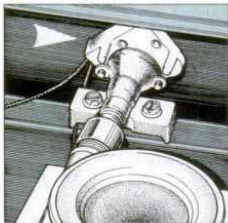
11 The black spot on this burner control switch (arrow) indicates the switch has been shorted and needs to be replaced.
