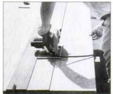
Position edge of guide on cutting line and clamp it in place. Now, make the cut. Keep the saw securely against guide strip.
