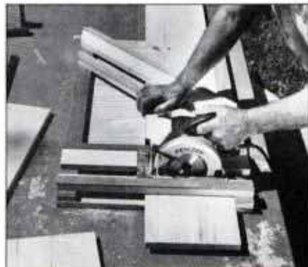
Track at end of jig makes accurate square cuts. Build jig to accommodate wide stock. This jig accommodates a 16-in.-wide board.
