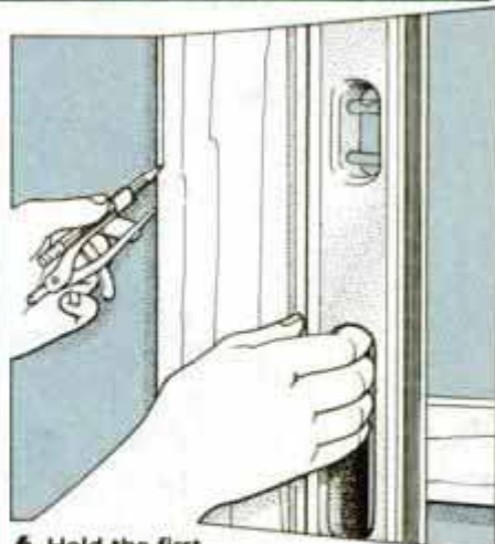
6 Hold the first piece of paneling plumb at the inside corner. Use a compass to scribe the board.
