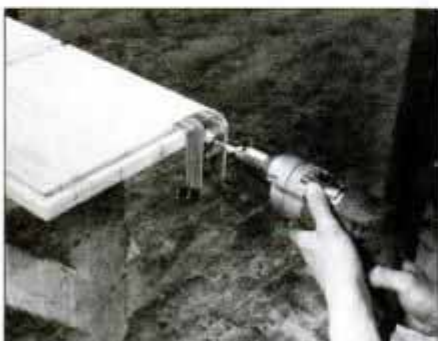
7 Bore \frac{1}{4} -in.-dia. \times \frac{3}{8} -in. dowel pin holes in top edge of each cabinet side. Use a doweling jig, as shown, to ensure accuracy.
