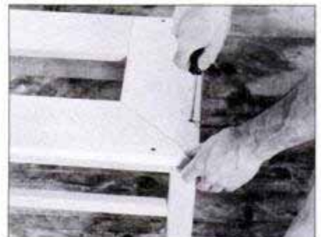
12 Position base frame over base so reveal is equal on sides and front. Then attach by driving screws through frame into aprons.
