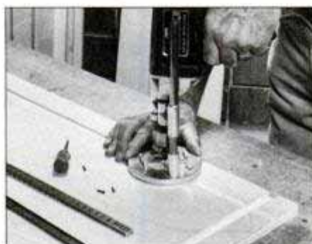
2 Cut standards to length, then bore pilot holes for their screws or nails. Do not attach standards until after finish is applied.
