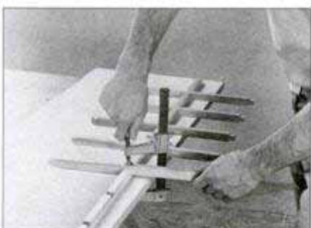
6 Apply glue to mating notches on grid parts, then bring each joint tight with a small clamp. Make sure assembly is square.
