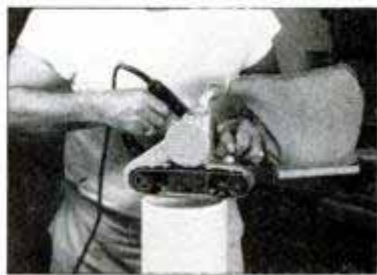
3 Remove saw blade marks from pipe ends with a belt sander. Keep sander moving at all times. Marks can be removed with a rasp, too.
