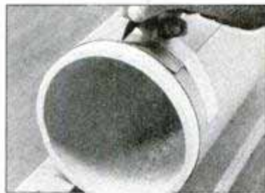
1 To ensure square leg ends, wrap a sheet of heavyweight paper around the pipe. Align overlapping edge and use it to mark the line of cut.
