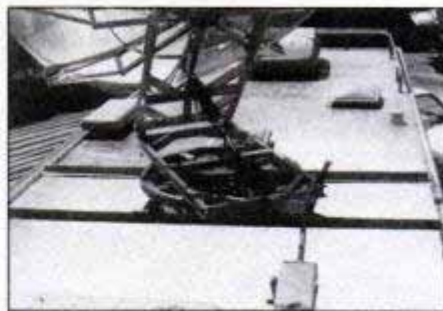
Dish, rotation and elevation mechanisms put great weight on an RV's roof. Wind loading adds stress. Horizontal aluminum bars (above) distribute the burden.
