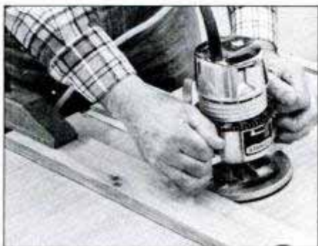
1 Clamp guide blocks to inner surface of cabinet sides and cut dadoses for web frames using a router and straight \frac{3}{4} -in.-dia. bit.
