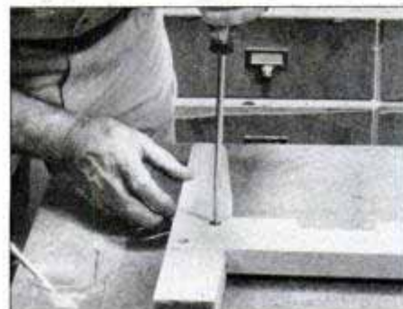
8 Assemble the glider frame with plastic resin glue and screws. Be sure to prebore screw pilot and 1/2-in.-dia. plug holes.
