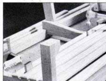
16 Insert 1/2-in.-thick spacer blocks between the seat slats to ensure even spacing. Set nails and fill the holes with putty.
