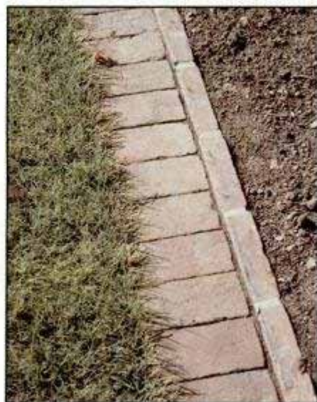
Brick sunk lengthwise on edge is mortared together to serve as a retainer for brick laid with long sides together.
