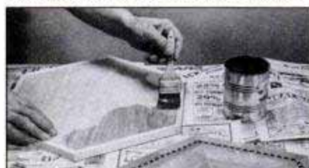
Apply veneer glue to the hexagonal assembly and to the table top which is made from ½-in. fir plywood edged in hardwood.
