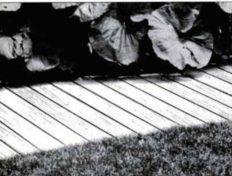
Wood 2x6s on sleepers separate lawn and planting bed, serve as a walkway when the lawn is wet and become a base on which the
