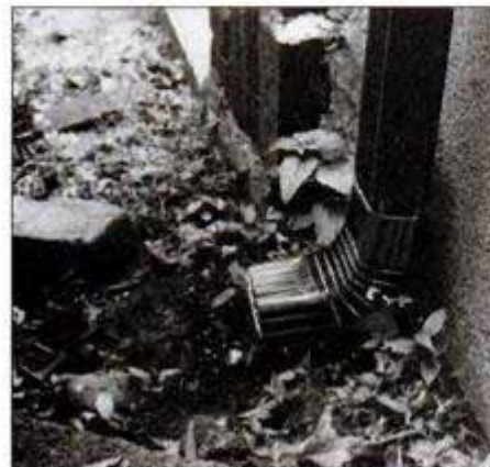
Problem 8: The base of this downspout should be extended, or a splash plate should be installed, so that water flows away from the house. Water from this spout had entered the basement.
