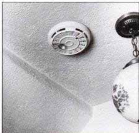
Problem 9: A fire hazard such as lack of smoke detectors is an easy and inexpensive problem to correct. A smoke detector should be located on the ceiling in the hall that is next to the bedrooms.
