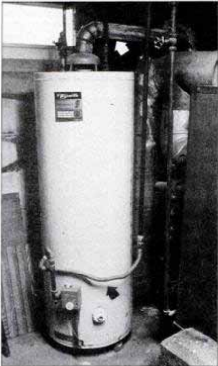
Problem 13: Incorrect installation of a water heater is a common occurrence. In this case the exhaust stack (white arrow) slopes improperly downward from the water heater to the chimney, and the gas pipe has a flexible connection (black arrow) rather than a rigid black iron pipe.
