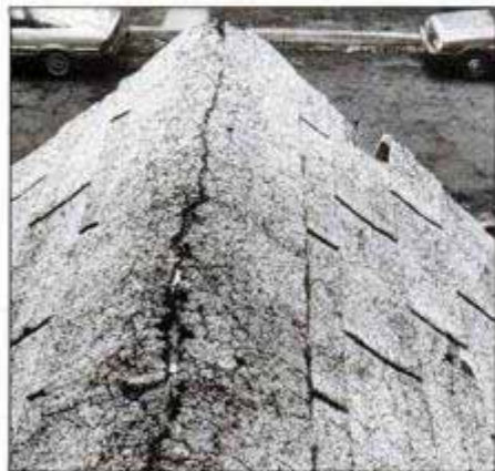
Problem 7: Cracked and deteriorating asphalt shingles are a widespread problem. These shingles on the roof ridge should be replaced even though there is no indication that water has leaked into the house.
