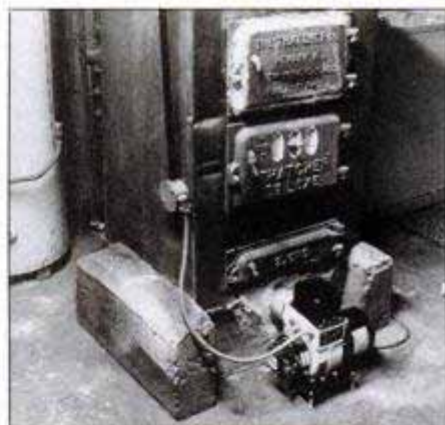
Problem 6: Antiquated heat systems are commonly in use. This old coal-burning boiler was made more efficient with a new oil burner (foreground). But there is no low water cutoff added.
