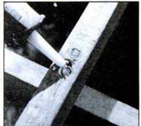
After tightening the beam-to-crossarm lagscrews, plug the counterbore with silicone caulking to seal out water.
