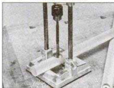
Mark stretcher locations on legs. Then, using a portable drill press attachment, bore holes with 1-in.-dia. spade bit.
