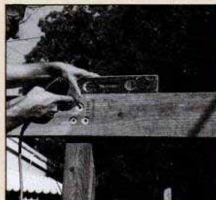
Hold crossarm level while boring pilot holes. Note that screw locations are counter-bored to accept screwhead and washer.
