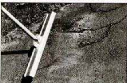
Patch potholes such as this caved-in chipmunk tunnel (top) with asphalt patch in a bag. Tamp the asphalt patch with a shop-made tamper to compact it. Patch cracks 1/8 in. wide or less with a liquid filler (above). Eliminate any tar stripes by sweeping some fine sand over the filler.
