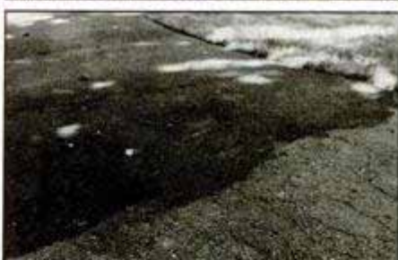
Cut away grass that grows over the edges of the driveway (top). Then sweep and hose away clippings. Brush the sealer completely to the edge of the blacktop surface. Use a tar base sealer with fine aggregate on worn asphalt (above, foreground) to fill cracks and smooth areas.
