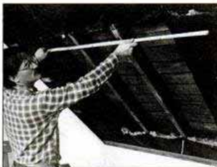
Choose window location inside room, then remove ceiling—in this case, pine boards—to expose rafter cavities. Measure across rafters to relocate window position.
