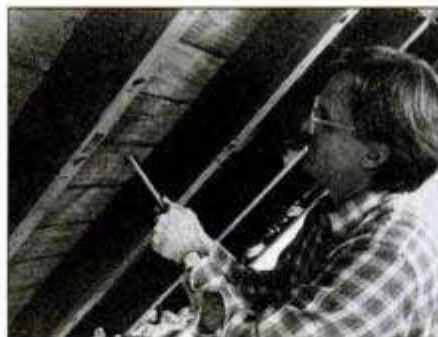
Bore hole through roof at centerpoint of desired window position. Then, slide dowel or piece of scrap wood into hole to act as measuring reference point on top of roof.
