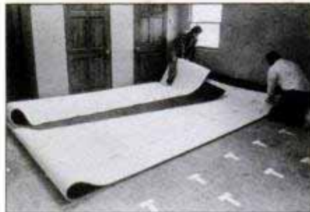
Position the largest piece of uncut carpet, folding as necessary. If possible, place finished factory edge at seam location.
