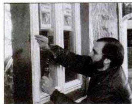
Plumb the window, then nail through the holes in the vinyl anchoring flange. Use large-head galvanized or aluminum nails.
