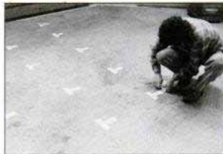
Tape down 6-in. x 6-in. Ts over the entire floor, spaced about 18 in. apart. Again, leave the protective paper in place.
