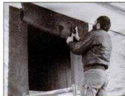
Staple 15-pound roofing felt around the rough opening before installation to deter air and water penetration.
