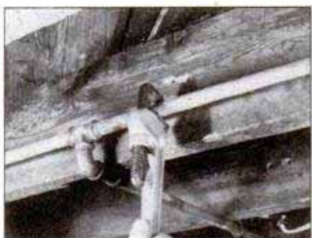
Tap into your existing cold water line by removing a section of iron pipe, as shown, or by cutting through a copper line.
