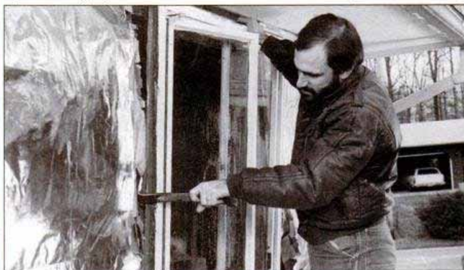
After loosening the old window from the inside, move outside and pull the unit from the house using a pry bar. This casement window was nailed through the exterior casing.
