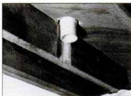
Place the waste flange in the hole and make sure it seats flat on the floor. Note how the joist side was cut slightly for fit.
