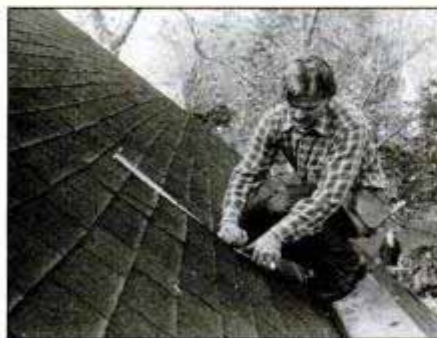
Hook tape on dowel to locate window, then draw rectangle on roof. Use a framing square for accuracy and check measurements from corners to eaves and ridge.
