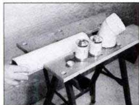
To join any fitting to the pipe, first wipe the pipe end and fitting seat with solvent and a soft cloth until both are clean.
