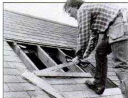
Pry off sheathing boards—or plywood sections, depending on roof—using flat bar or wrecking bar. Be sure to remove all nails from boards and rafters before proceeding.
