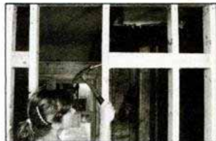
Nail 2×4 blocking flush to the inside edge of all studs on the rear and side walls.
