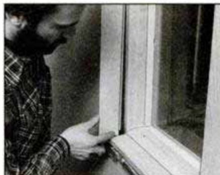
Fit the extension jambs into the window's prerouted grooves to build out the window jambs flush to the interior wall.
