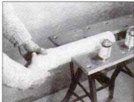
Slide the fitting over pipe and push until the pipe is seated. Then turn fitting 1/4 turn to make sure cement spreads evenly.
