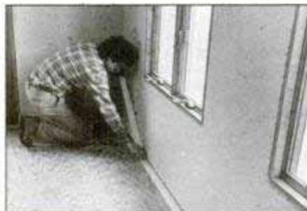
Remove baseboard, then run 2-in.-wide double-face tape around the room perimeter. Leave the protective top paper in place.
