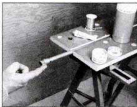
Allow the pipe to cool for several minutes—or dip it in water—then cover threads on the adapter with joint compound.
