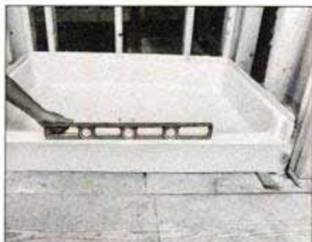
Center shower base in framed enclosure, then level all four sides. Install shims where needed, then trace drain hole onto floor.
