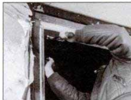
If necessary, frame-in the rough opening to accept the new window. Nail stock to the header first, then to sides, as shown.
