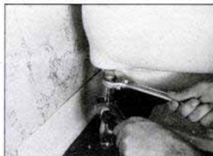
Make sure that all water is sponged from the interior of the storage tank, then remove the supply line and shutoff valve.
