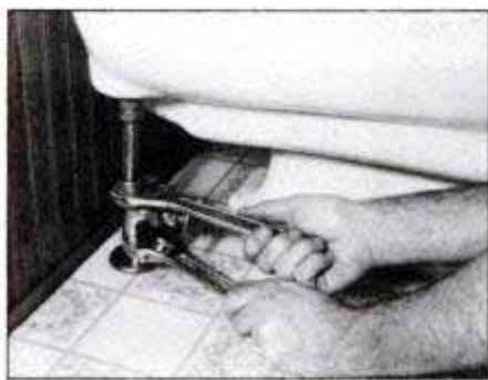
Reinstall the shutoff valve and join it to the toilet tank with its extension nipple and compression fitting. Turn on the water.
