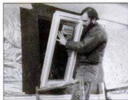
Place the new window into the rough opening, bottom first. Keep pressure against the sill while positioning the top.
