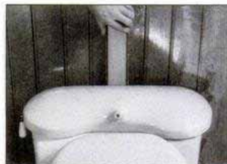
Center the bowl over the floor line, then push it against the wall with a piece of wall finish material held between the two.
