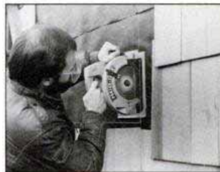
Snap chalklines from hole to hole to outline the window's rough opening. Then, use a circular saw to cut out the sheathing.
