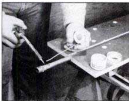
Using a propane torch, heat the joint with the tip of the inner blue flame. When hot enough, the solder will melt into the joint.
