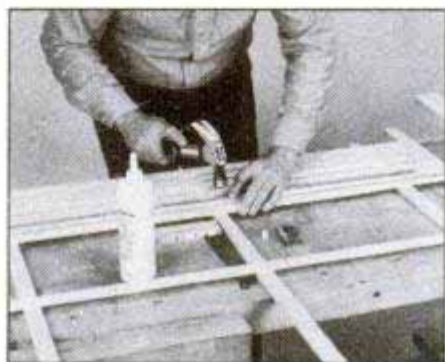
Place \frac{1}{2} -in. scrap between slats for even spacing, and secure slats with glue and \frac{5}{8} -in. brads. Keep slats square with the supports.
