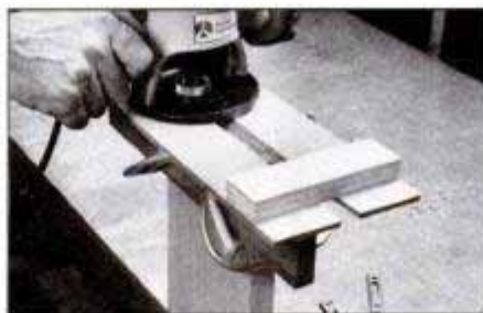
Mortise the rail ends with the aid of a platform jig. Space the plywood parts to accommodate the router's guide bushing.
