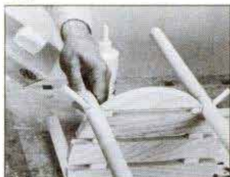
Bore holes for the dowel pegs with legs held at right angles to the shelf. Glue and tap dowels through the legs and into the shelf edge to complete the joints.
