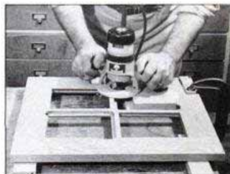
With the door clamped face down, rout out the back side of the sticking to permit installing the 1/8-in.-thick glass panes. Use wood blocks to support the router base.
