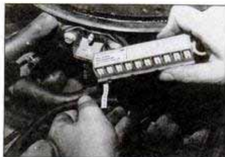
Numbered tape can help make labeling electrical connections an easy and neat job.
