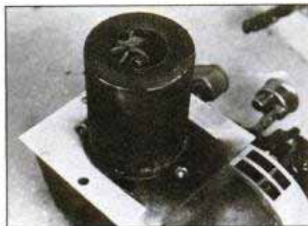
Clean soot from burner with wire brush and solvent. Then spray shroud and plate with high-temperature aluminum paint.
