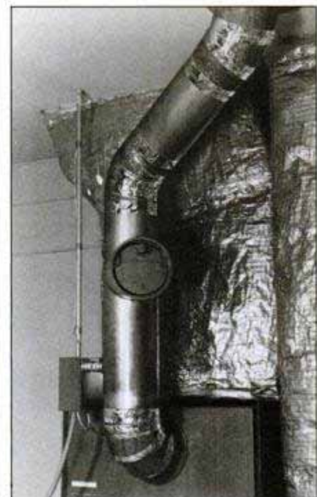
Replace old corroded galvanized flue pipes with new pipes that are made from stainless steel sheets. The joints should be sealed with 3M's metal repair tape.
