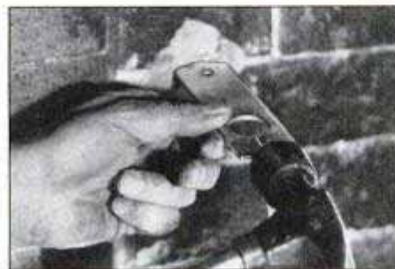
Indoors, toward the firebox front, install the bracket to hold the cable. Bore three 2 in.-deep holes spaced 3/4-in. o.c., apply epoxy resin and hammer the bracket in place.
