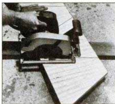
Cut the toolbox ends 1-in. oversized with a portable circular saw. Use a fine-tooth saw blade to prevent splintering the veneer. Move to table saw for final trimming.
