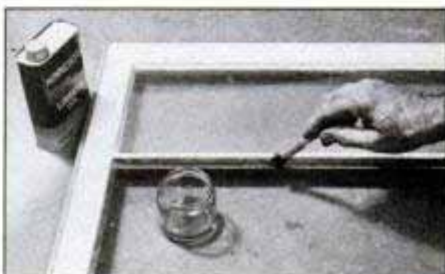
Apply a light coat of linseed oil to the bare wood so it will not absorb oil in the fresh compound. Otherwise, new compound will dry, lose flexibility and crack sooner.
