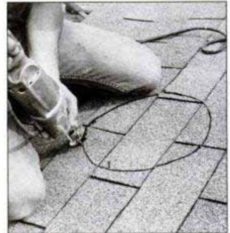
9 Pound four nails up through the roof to serve as guides for transferring the circle layout to the roof shingles.
