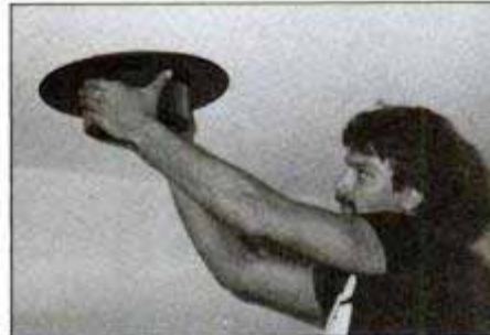
5 Lift the chimney support into place from below while your helper in the attic grasps it and positions it properly.
