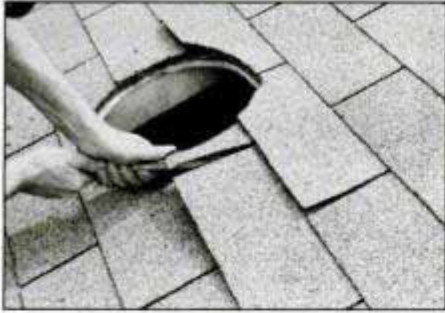
10. Loosen the shingles on the upper half of the roof cutout to facilitate the sliding of the roof flashing into place.
