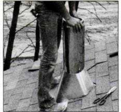
12. Insert a section of chimney through the flashing fixture and return to the attic to check for proper alignment and clearances.
