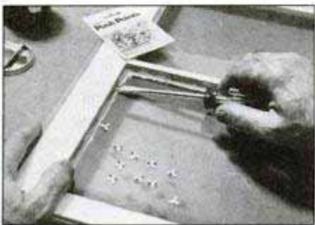
Secure glass with glazier's points pushed into the muntin and sash frame every 4 in. The push-type points shown are much easier to use than the flat triangular points.
