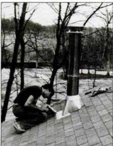
16. Seal shingles with roofing cement. Install rain collar. Seal it and the nailheads on lower flashing with silicone caulk.
