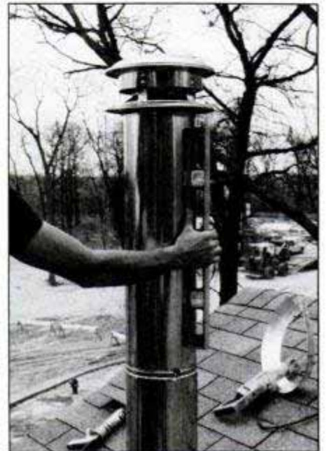
15. Add remaining chimney sections, rain cap and locking bands. Plumb the chimney, then caulk and nail the flashing.
