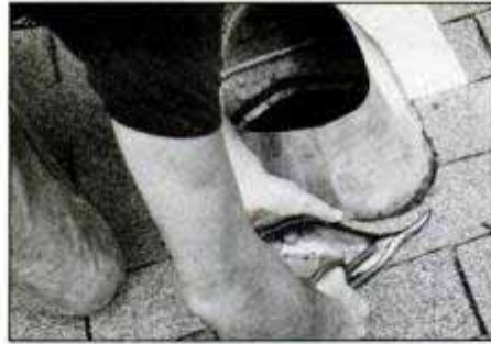
11. After sliding the roof flashing into place, you may have to trim the shingles a bit to center it on the opening.
