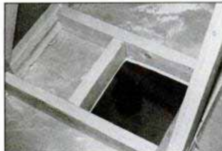
4 Working from above the finished ceiling, cut and install 2x4 lumber to bridge the joists and frame the opening.
