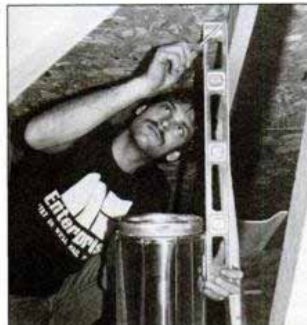
8 Using a level as a guide, scribe a circle at least 2 in. greater in diameter than chimney on roof deck's underside.
