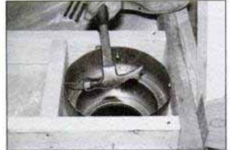
6 Have the helper in the attic secure the chimney support to the frame with screws or nails as instructions specify.
