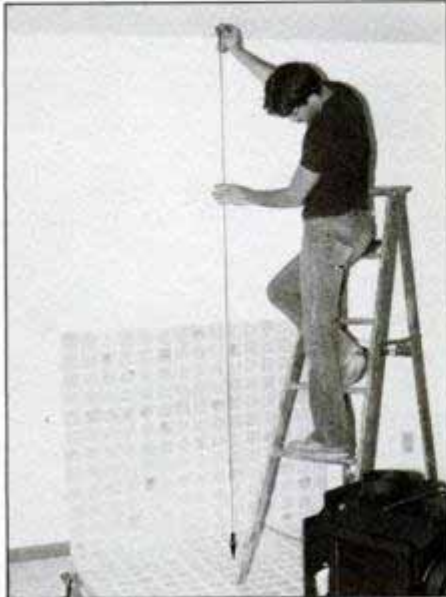
1 After centering the stove and marking the floor, drop a plumb line to find the desired ceiling penetration point.
