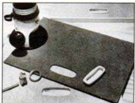
Rout the doors for the recessed maple pulls using a hardboard template, a 7/16-in.-dia. guide bushing and a straight bit.
