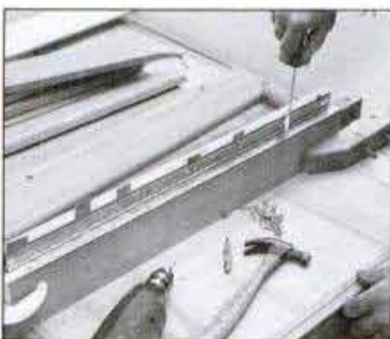
To position hinge, clamp the two mounting boards together with 1/16-in. shims between them. This method recesses the hinge below the seat surface.
