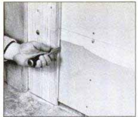
If board is slightly warped, you can often pry it tight by driving a chisel into the wall or furring strip and pulling back on chisel. Hold in place while driving nail.
