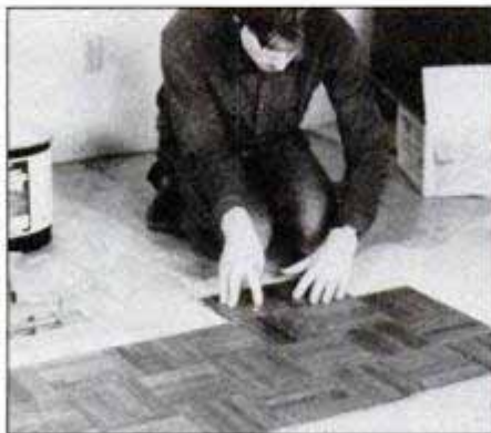
Follow the two worklines as you add tiles. Lay the second and third tiles on either side of the first one. Work from the center of the room toward the edge.
