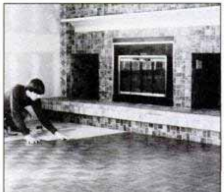
Work on a quarter of the room at a time, filling in the area between the two intersecting guidelines. You may have to trim the tiles to fit at the edge.
