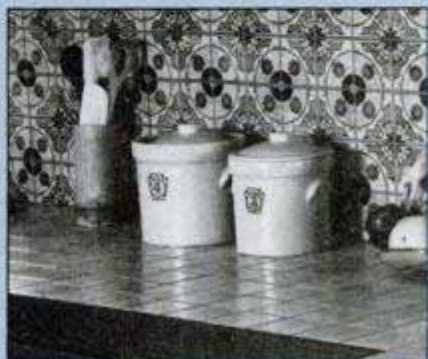
Apply grout and polish the tile using the same procedure that was detailed for the quarry tile floor. Let the work stand for 72 hours, then seal the grout.
