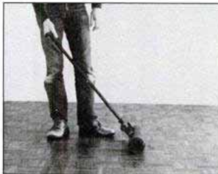
When the entire floor is laid, roll it with a 150-pound steel roller to ensure that the tiles make good contact with the adhesive and that they are level.
