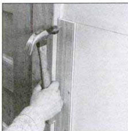
Once board is planed to fit, nail in place with finishing nails near back edge. The end boards are only ones nailed through surface. Set heads and fill holes.
