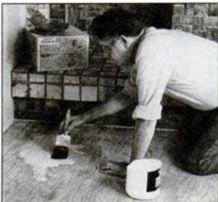
Old or new, prime the subfloors to ensure proper bonding with the adhesive. But before this step, drive in protruding nails, fill holes and nail loose boards.
