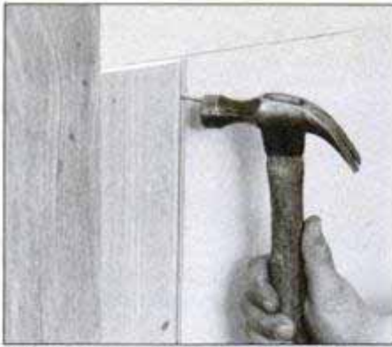
Attach tongue edge of board by driving nail through rear corner where tongue and bead meet. Angle nail at approximately 45° and set head.
