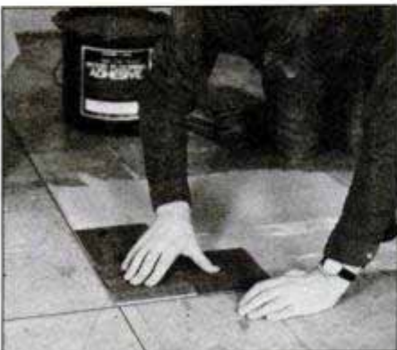
Set the first tile at the intersection of the lines. Be careful to align edges carefully with the working lines, since other tiles are aligned with the first tile.
