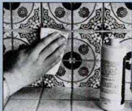
You can use an adhesive remover to clean the face of tiles before grouting them. Note that backing of the tile sheets is visible between tiles before grouting.
