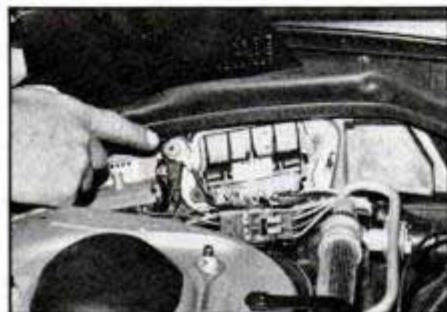
Master ground post for two-wire electrical system is located at Buick/Olds firewalls.
