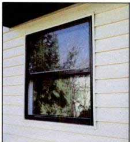
A close-up of the completed job shows almond siding with trim around the double-hung window, new soffit overhead.
