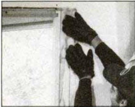
Install the finished headboard and seat-board by nailing through the extension jamb. Fill gaps at jambs with batt insulation. Don't force insulation into the spaces.
