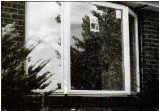
View shows unit without trim. To finish the top of the window, we screwed 2x4s into the rough head to serve as cleats. Then we installed 1/2-in. plywood flush from window flange to soffit.
