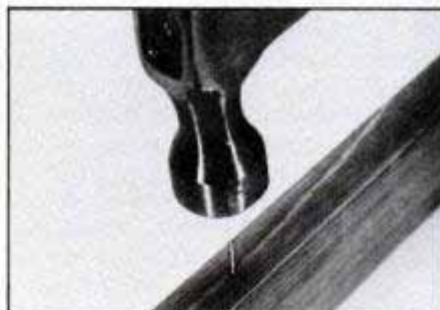
Space the nails as needed and drive them partially into the edge of the workpiece.
