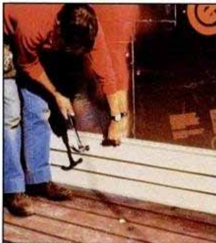
Siding is applied above the raised deck in the back of the house. Note that the seams of the rigid insulation are offset.
