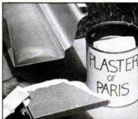
Seal end caps on the gutter with plaster of Paris to prevent chance of leaks.
