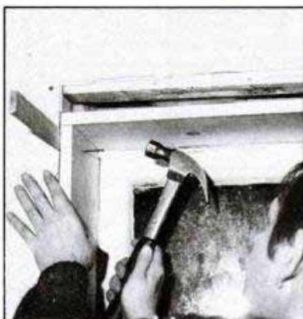
Use shims to hold the jamb in position for nailing. Be sure to check the jamb for square before you drive in the nails.
