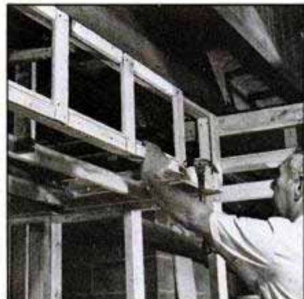
Last step in building framework is to nail filler blocks between vertical suspension boards. This provides necessary support for installing drywall corner bead later.
