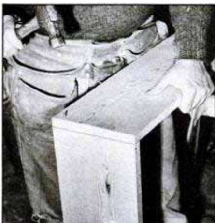
Preassemble the jamb before you nail it into the rough opening. You should use 2-in. finishing nails and simple butt joints.
