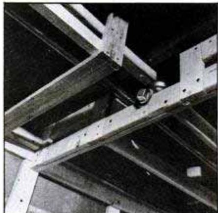
Don't cover up pipes or other obstructions that require servicing, such as the waste line cleanout plug above. Instead, scribe and cut framework so plug is accessible.
