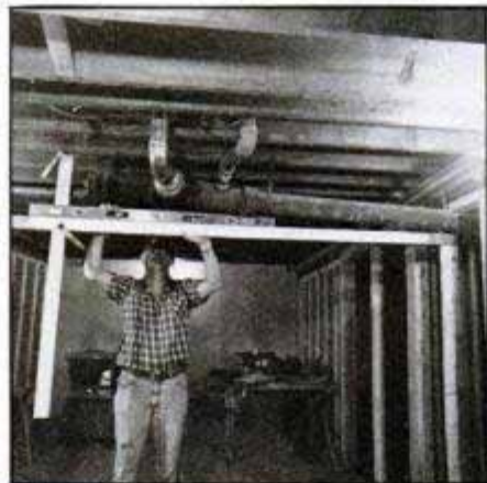
Tack-nail board to wall stud just under marked line and another board to floor joist, as shown. Clamp together, adjust for level and plumb, then mark for cutting.
