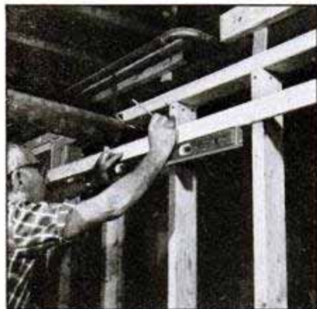
Begin framing by finding lowest point of obstruction (waste line above) and positioning a level furring strip at that point. Draw a line across studs at top of strip.
