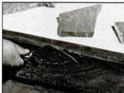
Fill the top form about half full. Carefully trowel mix into the cove of the form and place the rebars in position.
