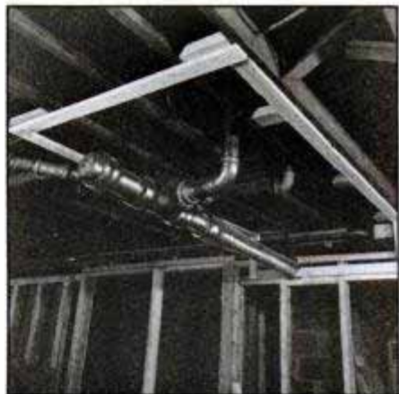
Install blocking between joists to provide sound nailing for frame boards. Then nail boards in place, making sure they're installed square to wall, even if pipe is not.
