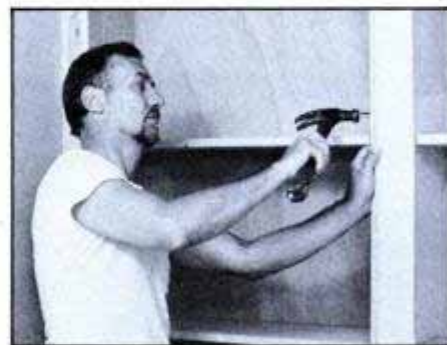
Use finishing nails to attach moldings to the interior edges of the stiles and headboards.
