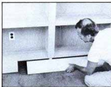
Two equal-length baseboards are used at floor. Electrical outlet plate mounts on back.
