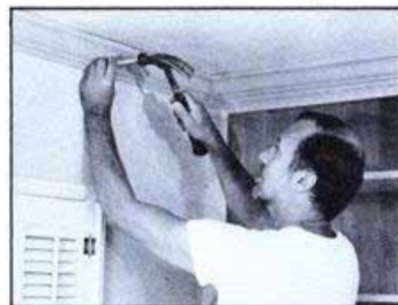
Extending the wide crown molding around the room completes the built-in look.
