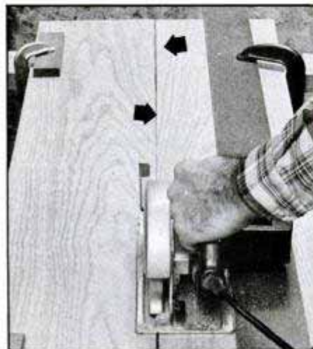
Steer the saw along a straightedge guide. Arrows indicate unevenness in board edges.
