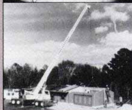
With a swing of the crane arm, Cardinal's house module moves from truck bed to foundation. Patented system allows the module to be lifted by its ridge pole.
