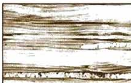
Grub holes bored by insects while tree was alive weaken and mar finished board.
