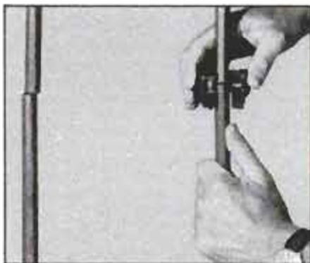
To begin installation, turn off the water. Then cut through the water-supply tubes leading to the old faucet. If floor-supplied, make the cuts at least 24 in. below the sink. Here, a close-quarter tubing cutter makes neat work of it. You can also use a hacksaw. Threaded supply pipes should be cut and unthreaded at the joint. (Drain parts and trap are removed for photo.)
