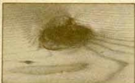
Unsound knot has surface damage, but it's tight and weakens timbers very little.
