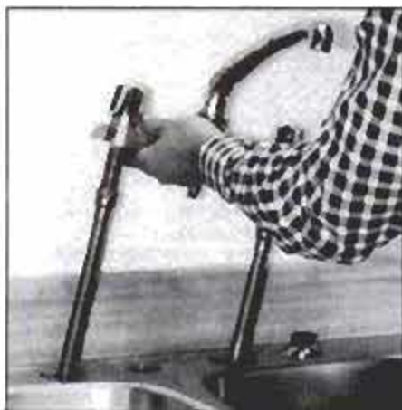
Remove the attaching nuts and washers under the old faucet and lift it out. This one has a female pipe adapter hook-up without shutoff valves or riser tubes. Copper tubes went from the floor slab to the faucet.
