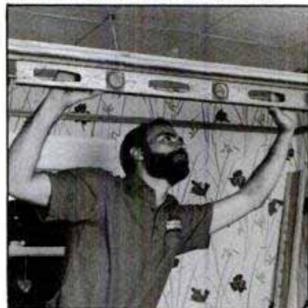
Check main beams for level after installation. Note that hanger wire passes through a hanger clip. Prevent wires aid positioning.
