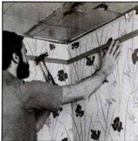
Snap a level chalkline to indicate ceiling height. Then, nail oak side rail in place. Pre-bore rail to prevent chance of splitting.
