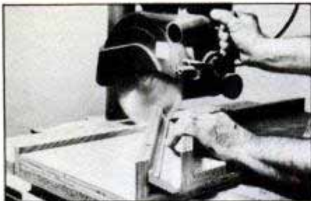
Cut tricky compound-angle miters in crown, bed and cove moldings with a radial-arm saw. The jig holds the molding at same angle as it's installed for accurate cuts.
