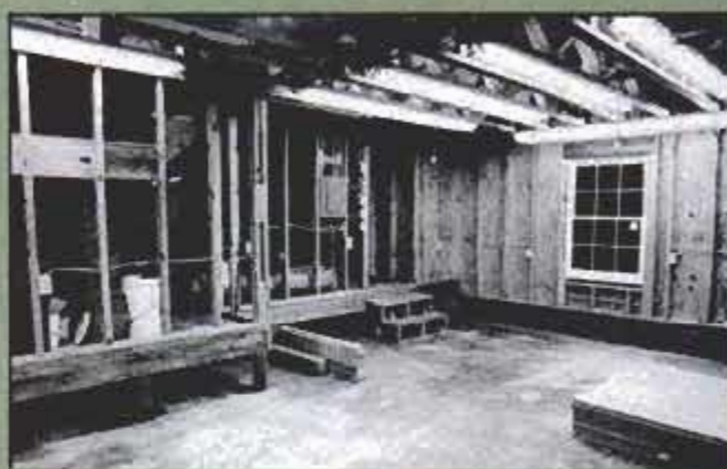
Photographs showing wiring paths on all sides of the room were taken for reference, should work on the walls be done later.
