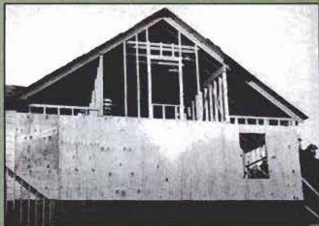
The 2x4 wall framing is almost complete. Anchor bolts spaced every 8 ft. in the masonry secure the mud sill to the slab.
