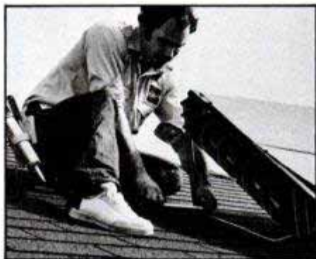
Parts for clamping the brackets come with kit. After boring pilot holes in roof sheathing, lagscrews are installed.
