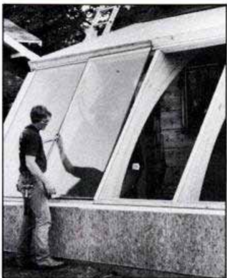
The 46 x 76-in. double-thick insulating glass panels are laid into the frames that are formed by the glazing stops.
