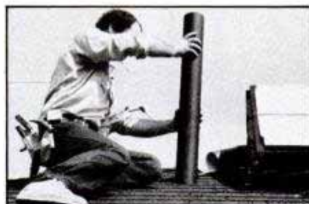
Duct hole is cut out with sabre saw. Then, the duct is positioned to mark the floor.
