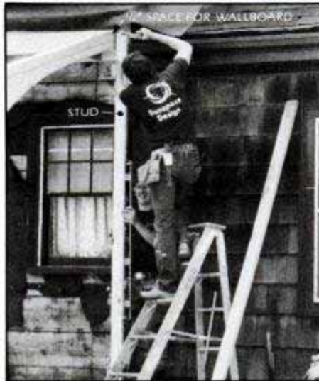
End-wall framing is completed by adding toeplate (not shown) and a vertical stud. Kit is being attached to the roof overhang, which provides extra room depth.
