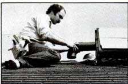
An elbow is fitted to a length of duct and exact location for duct cutout is marked.
