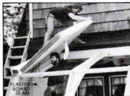
Roof panel is being set in place. Note that plasterboard on inside of end wall will need finishing only at the seam.
