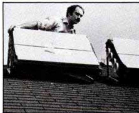
To join two or more units, the knockouts along mating sides are removed and units are coupled using short pipe lengths.
