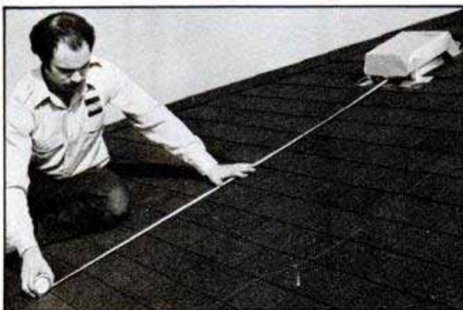
First step on the roof: Use a tape measure to lay out for the most pleasing plate appearance and efficient duct run.
