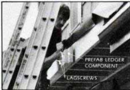
A ledger is attached to existing structure where the beams will join. Rabbeted end strengthens joint between the sections.
