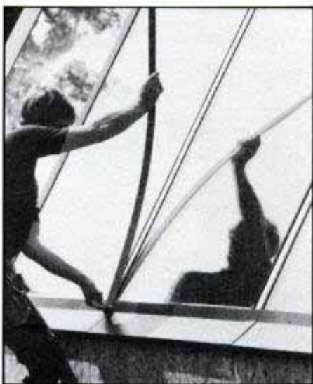
Finished sheet-metal flashing is pre-cut and prebored for fasteners. Caulk flashing edges with clear silicone.
