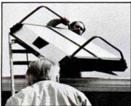
Panels are lightweight and easily transported up ladder by one man, then handed to work partner already on the roof.
