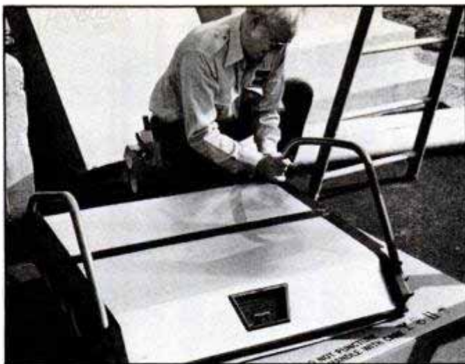
Panels snap together in minutes. Most assembly is done at factory. Here, designer Jack Hanson installs the second bracket.
