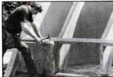
Wooden block is used to prevent damage to kneewall panel as it's forced into place. Corner component is visible at left.
