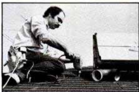
Using an extra-long drill bit, a hole is bored through at exact center of cutout.
