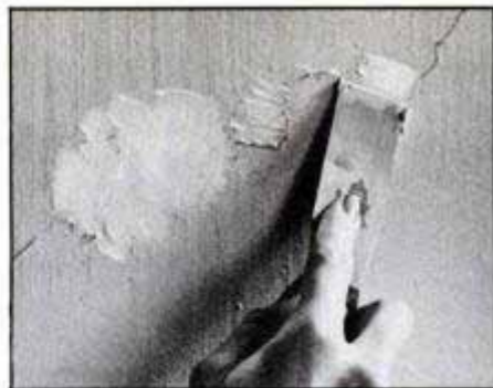
Above shows how not to apply joint compound over cracks—unless you want to do a lot of sanding. Don't dab it on; apply a smooth coat with wide-blade knife.
