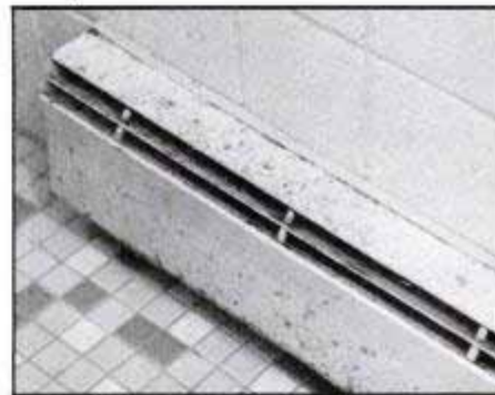
For a perfect finish, remove all paint from peeling baseboard heater housing, then apply the primer and finish coats.
