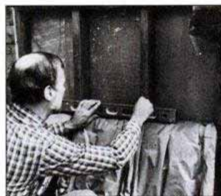
On studs under window, mark position for header and sill. Dimension is height of air conditioner case plus two 2×4s.
