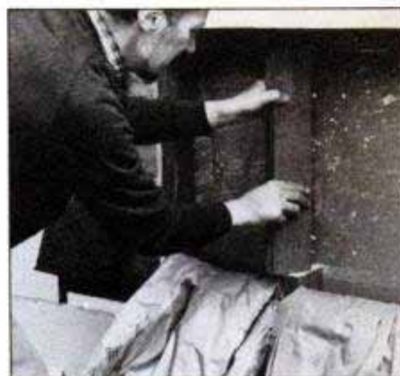
Section of cripple stud is removed after sawing out. Pull away from plasterboard.
