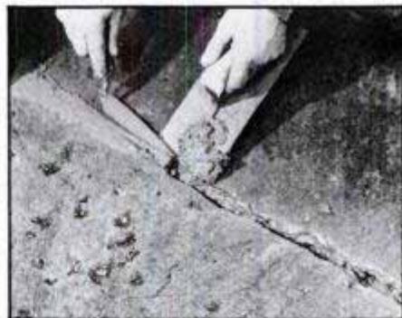
Fill the crack with a patching mixture of portland cement and sand or vinyl patching compound. Poke material deep into the crack with the trowel point.
