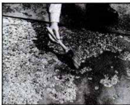
We applied a liquid bonding agent to the floor for good adhesion of our sand-cement patching mix. Vinyl patching materials don't need bonding agent.
