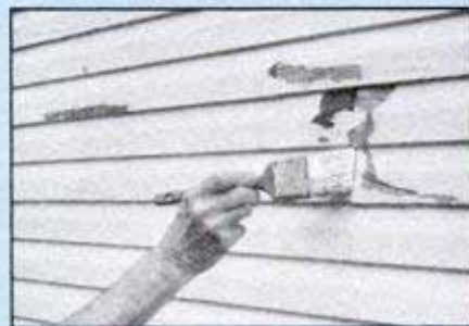
Step 3: Allow glue to dry 24 hours, and then apply primer suited to topcoat.
