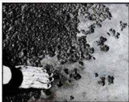
Pitting and spalling shown here were caused by de-icing salts. To prepare for patching, clean away residue and dirt by brushing and flushing with water.
