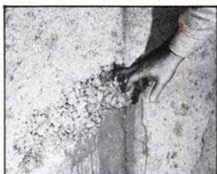
This air pocket, or honeycomb, was formed at the time the basement wall was poured. Structurally weak, honeycombing may be source of water leaks.
