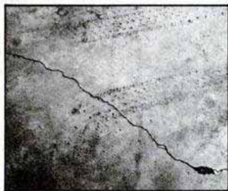
Narrow cracks, like this one in a concrete garage floor, can be patched with a vinyl polymer compound available in tubes.
