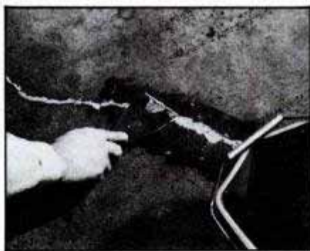
Run a bed of patching material over crack, using a caulking gun. Press compound into crack with a moistened putty knife and let it set about 15 minutes.
