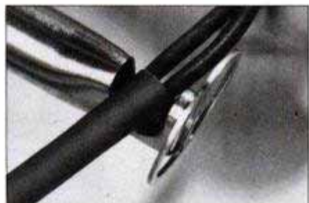
Slip a third piece over the "trunk" and overlap the two previous pieces of tubing by at least \frac{1}{4} in. Apply heat.
