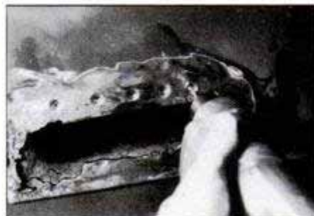
Drill \frac{3}{32} -in. holes into the center of the dimples. Make sure holes are centered or screws won't be flush with the metal.
