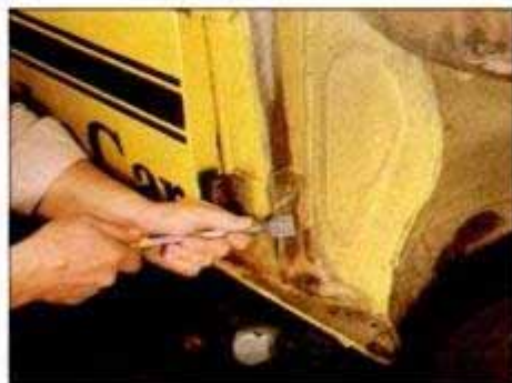
Loose scale can be removed quickly with a gasket scraper. Get off as much as you can before going to the wire brush.
