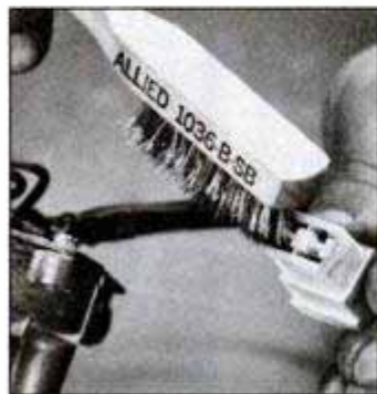
Corroded spade lugs in connector should be cleaned with wire brush. If it is necessary, resolder the wires.
