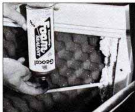
In areas hidden by trim panels, expanding foam urethane provides temperature and sound insulation. Use it sparingly.
