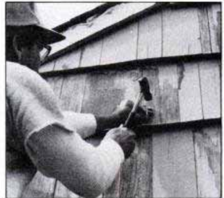
Secure loose siding by face-nailing it with galvanized nails. Replace siding that's rotten or damaged beyond repair.
