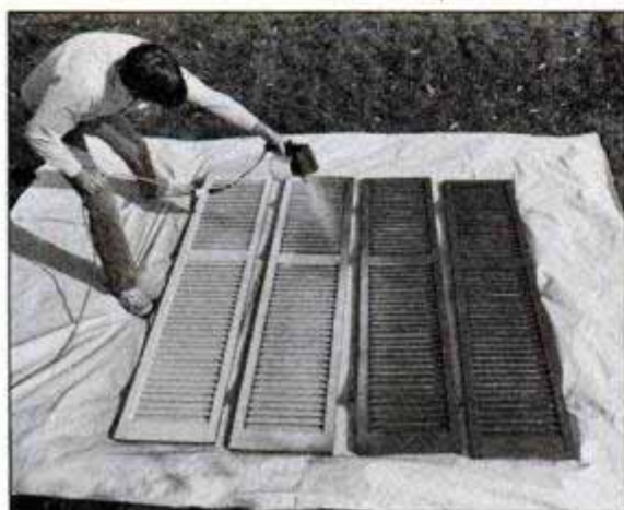
Shutters were laid flat to reduce the chance of paint sag and drips. We numbered the backs of the shutters to keep track of where they came from and replaced them using the same nail holes.
