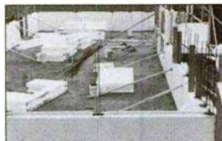
The walls are 12-in.-thick foam blocks coated on the outside with Insul/Crete.
