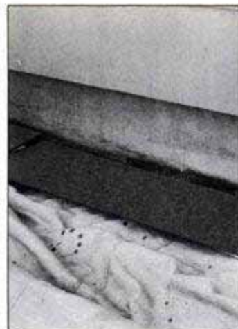
Strips of hardboard or scrap come in handy for holding down dropcloth edges. Space them 1/2 in. from foundation.
