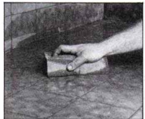
14 When the grout begins to set (30 to 60 minutes), clean any excess from the tile surface with a damp sponge. Rinse sponge often with clean water.
