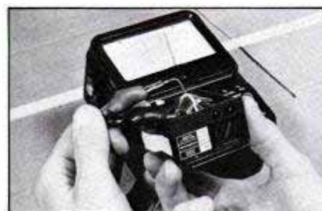
8 Test motor for continuity by placing probes across the two motor leads.
