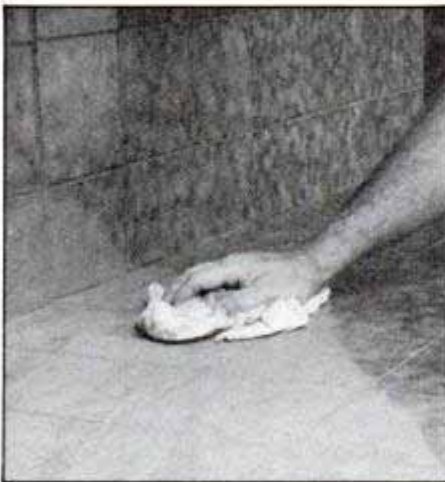
15 Allow grout to dry thoroughly. The grout residue remaining on tiles can be cleaned off with a soft, dry cloth.
