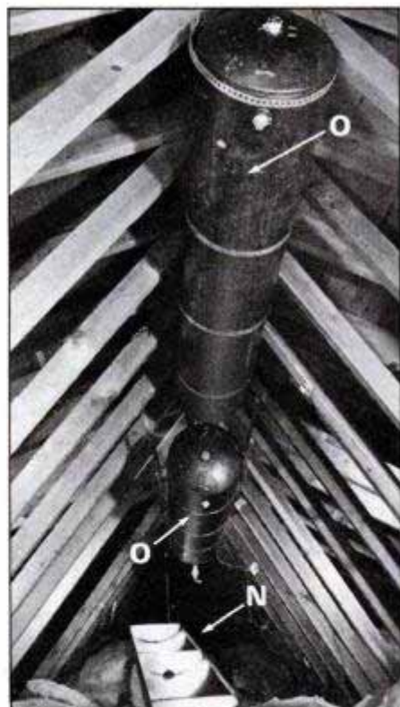
Tempering tanks (O) have 30-gal. capacity each and are hung from roof trusses or rafters with perforated metal strapping. The condensation tray (N), which drains to the outside, is a safety feature.
