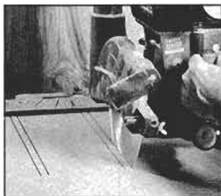
Parallel cuts halfway through panel form the deep edge half-lap notches. Use chisel or sabre saw to drop out waste.
