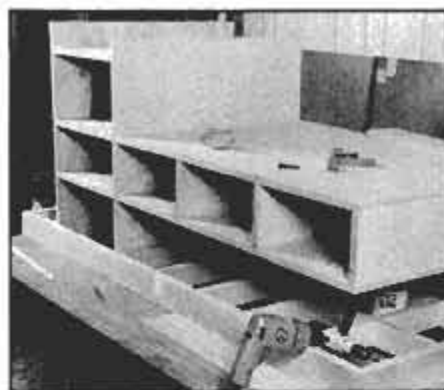
View shows how a drill equipped with a right-angle drive is used to bore the lag-screw holes in this tight spot.
