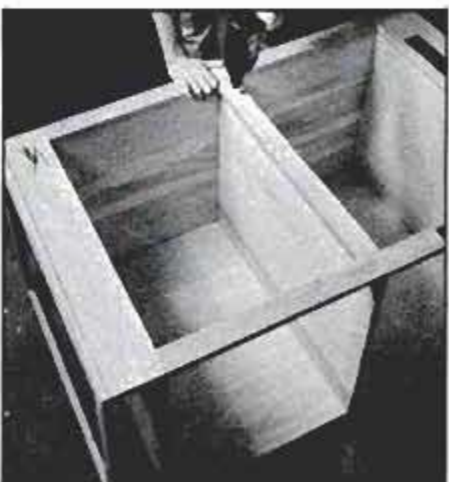
To attach facing, bore pilot holes to prevent splitting and to keep nails from bending due to the ash's hardness.
