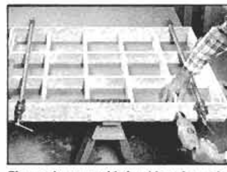
Clamp the assembled grid to bore the screw body holes into the cross members. For accuracy, you can use a square.
