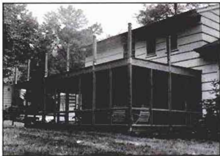
Framing of the lower porch is complete. The railing posts on the upper deck are in place and the roll roofing has been installed.
