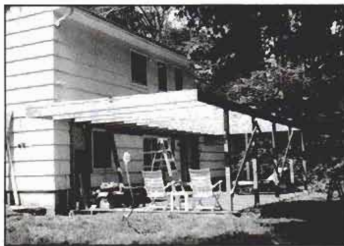
Support posts and joists have been installed in this view. Note the temporary diagonal bracing on the posts during framing.
