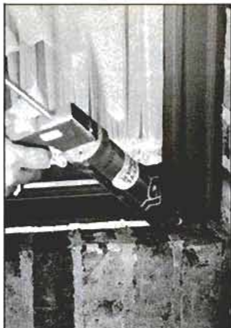
Metal frame for sliding window should be caulked by pushing gun (from left to right as shown here) to force caulk into crack. Push gun; don't pull it toward you.
