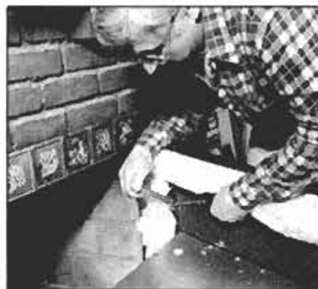
With trim pieces installed, machine screws can be turned home using a pliers. Slot in the foreground is the unit's damper.
