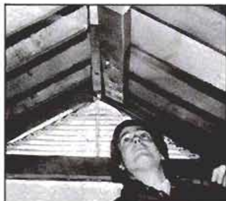
Inside, a 2x4 cleat is spike-fastened across several rafters; upper brackets are anchored to this member, while another is installed near eave for lower brackets.
