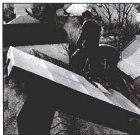
Panel is large and heavy enough to require two men to do the hauling up to the roof.
