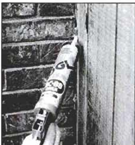
Sealing a vertical joint where brick chimney meets board-and-batten siding keeps out driving rain. Push the gun up at an angle to drive caulk deep into cracks.
