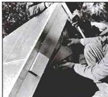
Correct tilt angle for the collector is determined using method that is described in the text. Once tilt angle is achieved, the support legs are then marked and cut.
