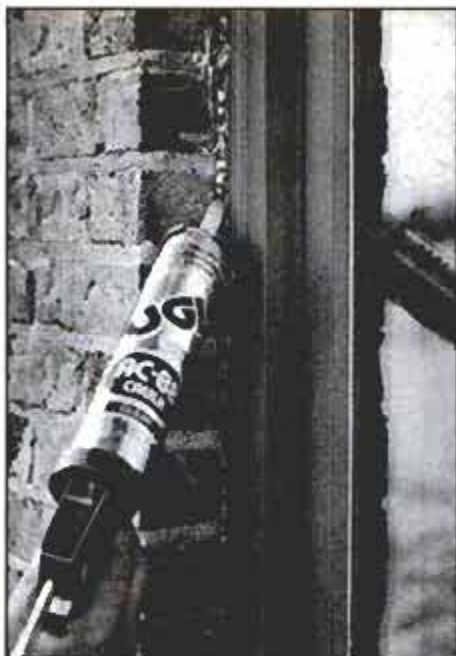
Caulk wherever unlike materials meet, even if you cannot feel an air leak or spot water seepage after a heavy rain. Here, wooden door jamb meets brickwork.
