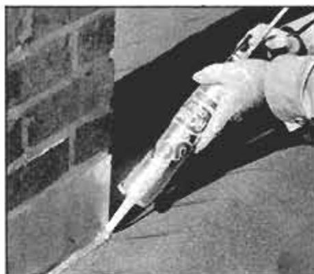
Black caulk is inconspicuous where metal chimney flashing tucks under the shingles.
