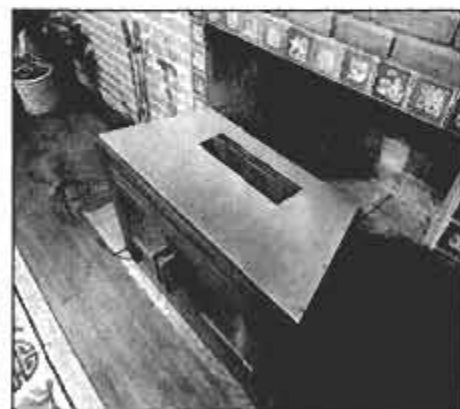
Insert is uncrated and set in front of fireplace opening. Since it weighs about 150 pounds, the job is easier with a helper.
