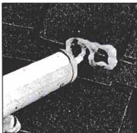
To prevent water leaks, quality caulk is applied and bracket is fully seated in it.
