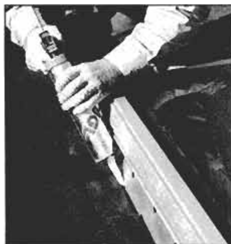
Push caulk into joints where a skylight meets the roofing and over the flashing.
