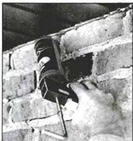
Aluminum-sheathed soffit meets brick wall and air escapes. Use dark caulk, match soffit color or use clear caulk which takes on appearance of adjacent surfaces.
