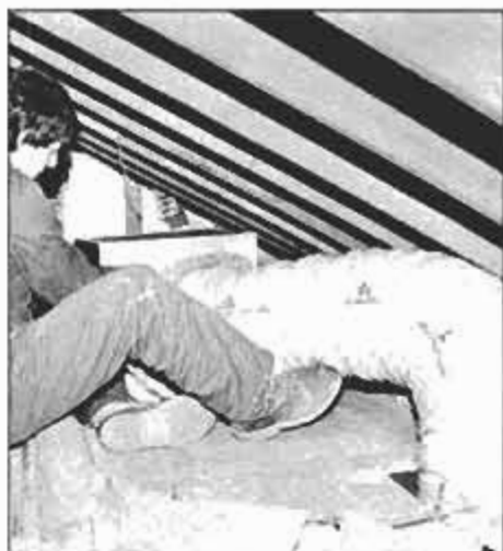
In attic crawlspace, Nelson Dina completes the hookup of the return air flexible ducting.
