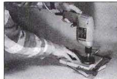
5 Prebore screw holes in leg wing, then cut concave arc with hole saw. Block clamped to wing provides center for saw.
