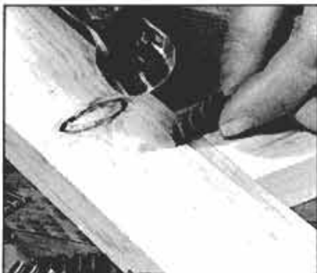
Hold butt-joined boards securely together—with clamps if necessary—while you drive wiggle nails. Author prefers to start one end in one board, as here.
