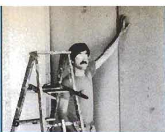
The final two construction steps show: 4. Notches being cut in the paneling for electrical outlets; 5. Particleboard being installed and prepared for the two coats of primer and two coats of semigloss paint.
