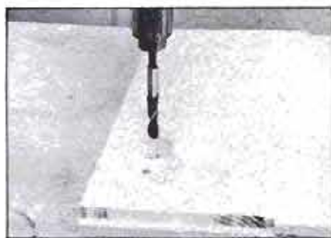
10 Bore blind dowel holes on marked sides. Check stop often; don't bore through.
