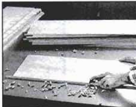
1 Use a block plane to trim edge banding flush with panel surface, then sand surface.
