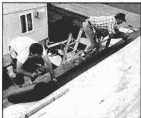
Next, lay 15-lb. asphalt-saturated roofing felt. Apply drip edge under the felt along eaves; over the felt along the rake.
