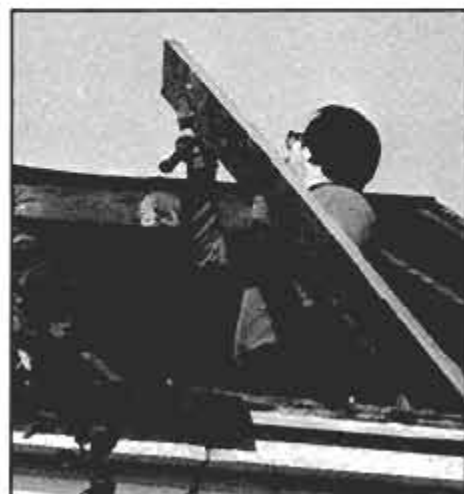
The two warped and twisted rafters should be removed and replaced with new ones.
