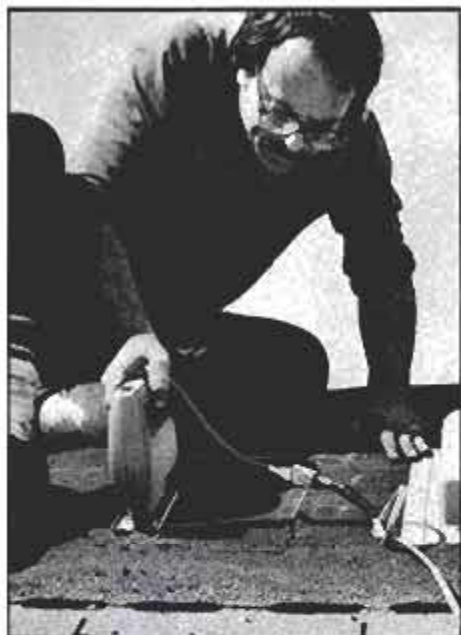
You should use a sabre saw to cut holes through the underlayment and the decking that's needed for the ventilators.
