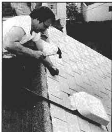
Here the final course of shingles is being applied to the first side of the roof.
