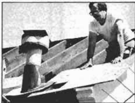
Carefully measure and cut the decking to custom-fit around the soil stacks, protuberances and other openings in the roof.
