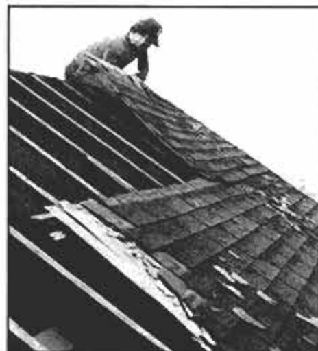
Pry all the rotted areas of the sheathing loose with a crowbar. These large sections of damaged roof must be removed.
