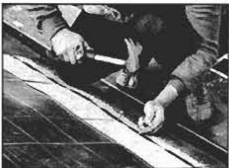
The starter strip is a row of inverted shingles which is covered by the first course of shingles. The starter strip seals the first shingle course.
