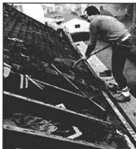
In areas where the sheathing is still serviceable, simply remove the damaged shingles with either a flat shovel or spade.
