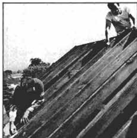
After all damaged sheathing has been removed, measure area to be covered carefully, so new panels are cut for neat fit.
