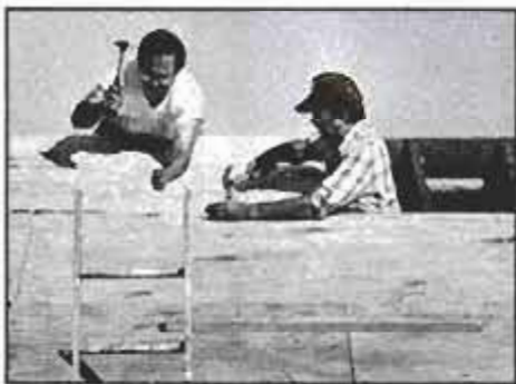
The ladders should be long enough to extend 3 ft. above the edge of the roof. In the photo, the next-to-last decking panel is attached. The decking panels are staggered to avoid long vertical seams.
