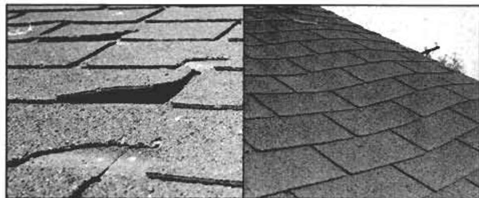
Overage shingles on this 37-year-old roof are curling, peeling and shedding granules. The brittle corners are breaking off.
