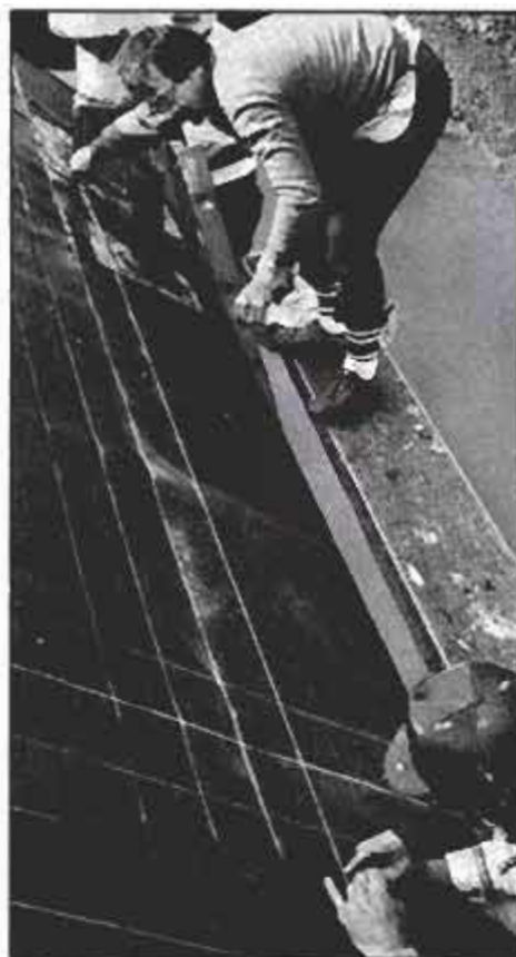
Snap chalklines at measured intervals to guide you in applying the shingles. Mark 5½ in. from the edge of the rake; then snap lines vertically at 6-in. intervals. Snap horizontal lines every 5 in. parallel to both the ridge and the eave.
