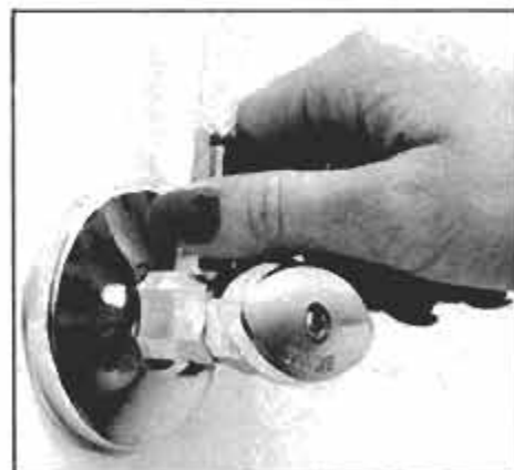
End of flexible tubing goes directly into compression fitting on shutoff valve.
