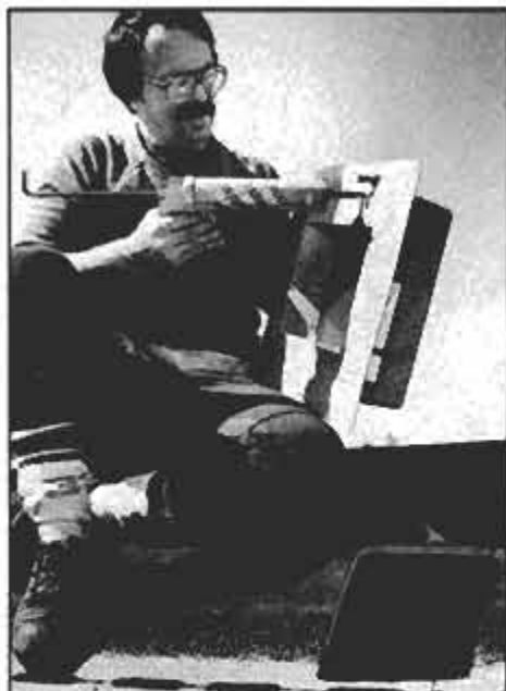
Seal the flanges on the vents and around chimneys thoroughly, using black plastic roofing cement in a cartridge-type gun.
