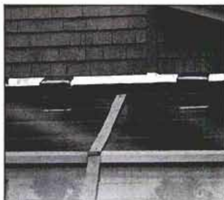
Double roof vents draw off warm air from the greenhouse by convection. Both are sealed in the winter to prevent heat loss.
