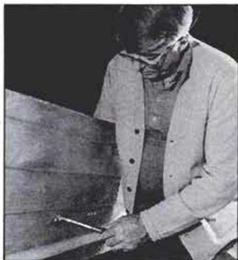
Small holes are fixed with Pliobond-coated aluminum patches held with Pop rivets.
