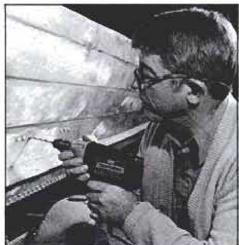
Loose rivets are drilled out and replaced with aluminum bolts, washers and nuts.
