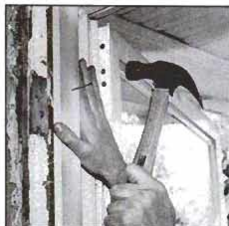
4 Nail furring strips to an unrabbeted jamb. The outside edge of the new door frame then abuts these strips (stops).
