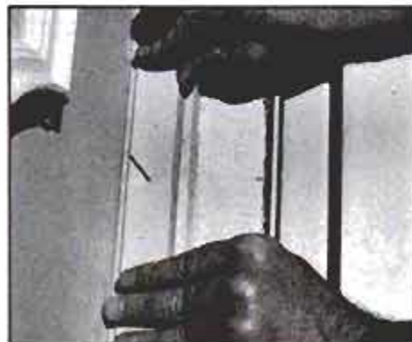
10 Nail weatherstripped stops (provided in kit) over furring strips with stripping compressed against door face, as shown.
